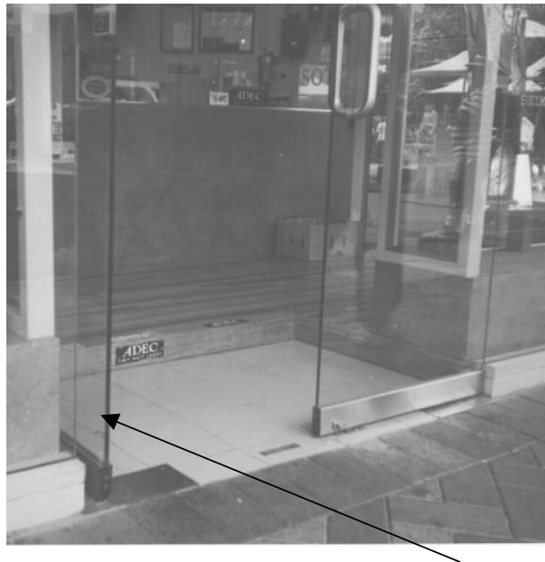
The false floor prevents access and the doors are less than 960mm in width
