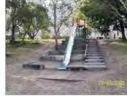
Playground equipment without any type of soft fall layer or other modern safety features. This equipment whilst still popular doesn't meet the latest safety standards and should be scheduled for removal and replacement.
