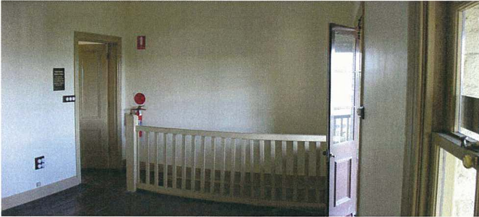
Figure 47: Room First Floor The staircase is reconstructed based on 1978 sketch drawings. Its pitch exceeds BCA requirements. Walls have been plastered over render finish. Dividing wall on left is studwork and plasterboard widened to represent a masonry wall thickness.
