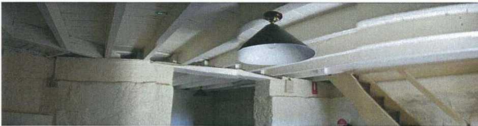
Figure 49: View of Lower Ground Floor ceiling of open joists and exposed butted boards. Timber joists and flooring painted to represent lime wash finish.
