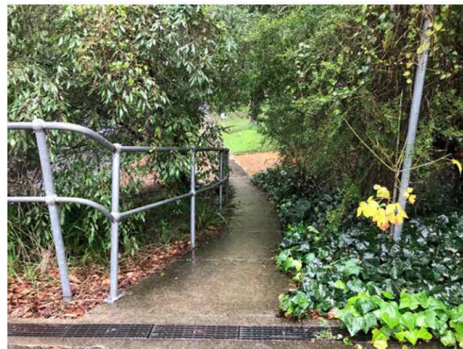
Non-compliant access from Epping Road
