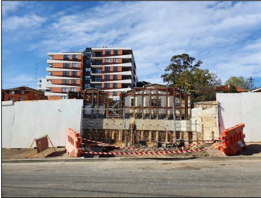
Figure 2 – View of site from Coulter Street depicting excavation and shoring works being undertaken and the rear of the existing Western Crescent facade
