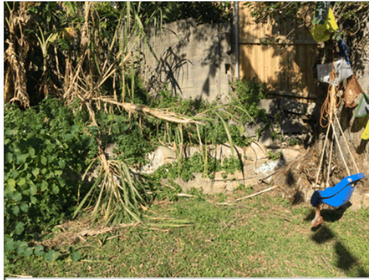
2324 - View east at front SE corner of No.101, 1.8m(+) high block retaining wall on boundary with No.103
