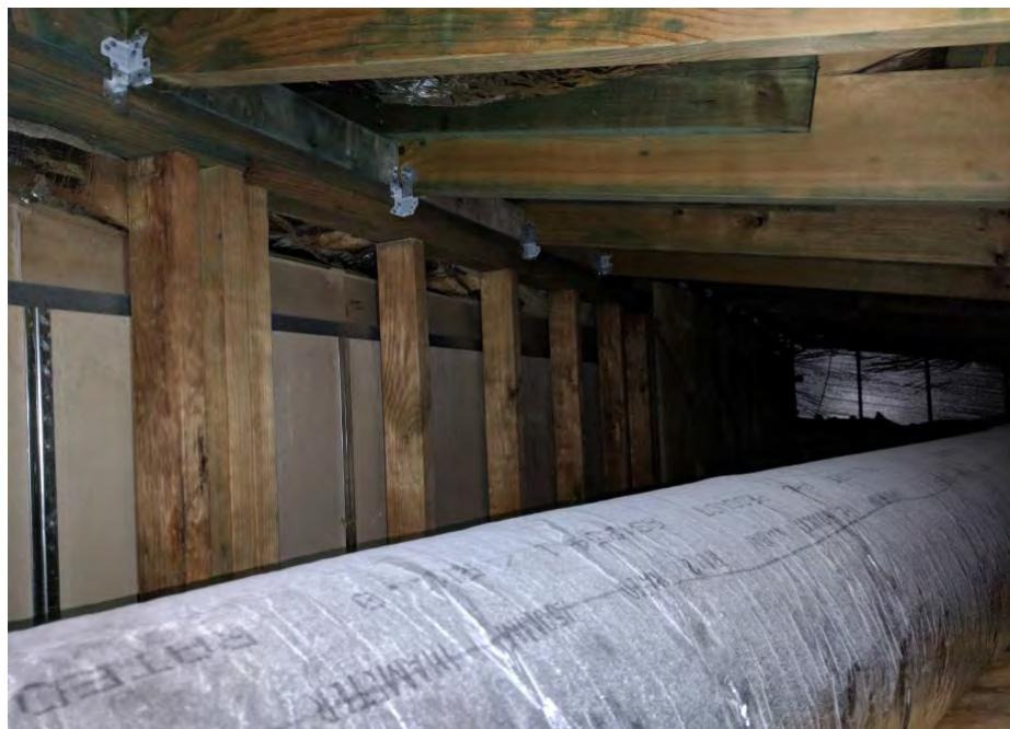
Figure 8 – Party wall within the roof cavity showing an apparent continuation to the ceiling in anticipation of conversion of the dwelling house to a dual occupancy (attached) building.
