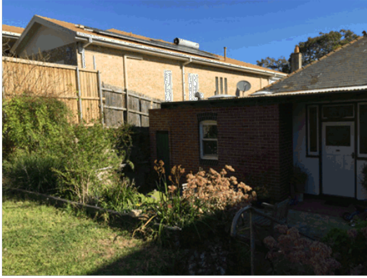
2323 - Front of dwelling No.101, view south to area of excavation for additions
