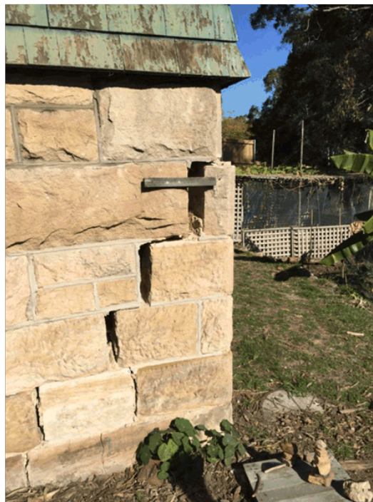
2306 - Footing settlement, wall rotation and displacement at rear corner of dwelling. Note sewer manhole at base of wall.
