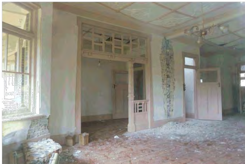
Figure 55: View of wall between loungeroom and hallway (foyer). Note the damage to the wall plaster is a result of illegal building works which occurred prior to the IHO on the site.
