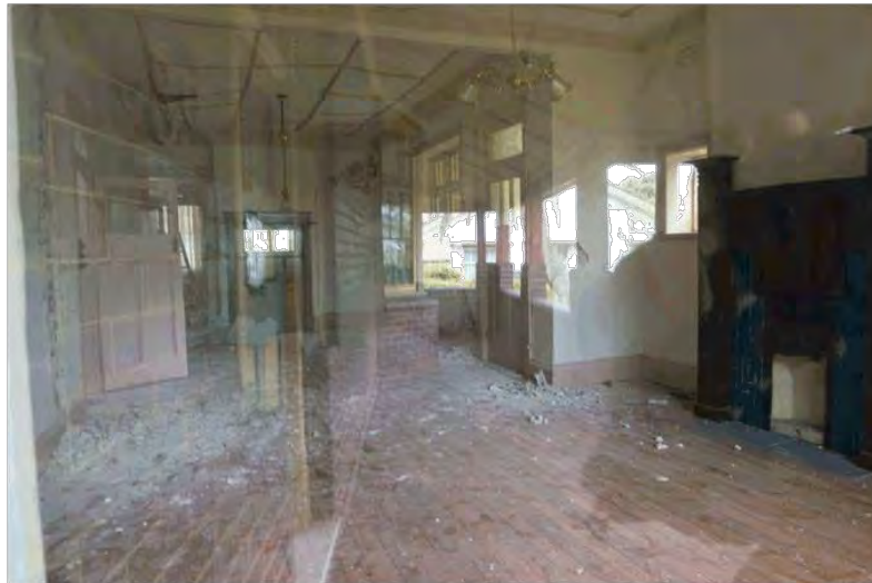
Figure 54: View of loungeroom and dining room looking towards the rear from front bay window
