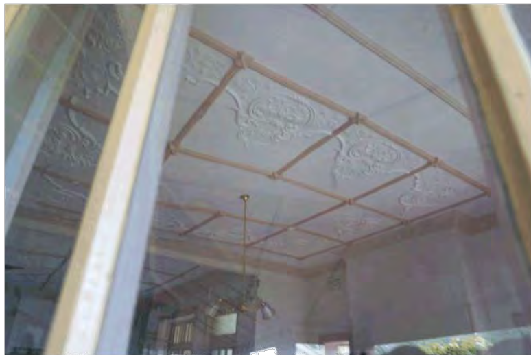
Figure 53: Lounge room ceiling, taken through front bay window
