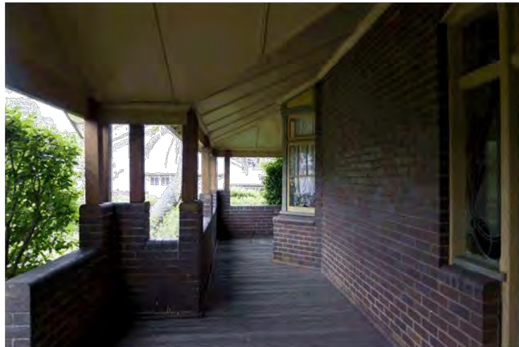
Figure 23: View along front verandah to the west, showing complex ceiling form and bay window
