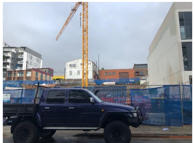
Figure 3 – Pre-construction photograph of the site from Farm Street looking north-north-east (with 11 Farm Street on the right of the photo).
