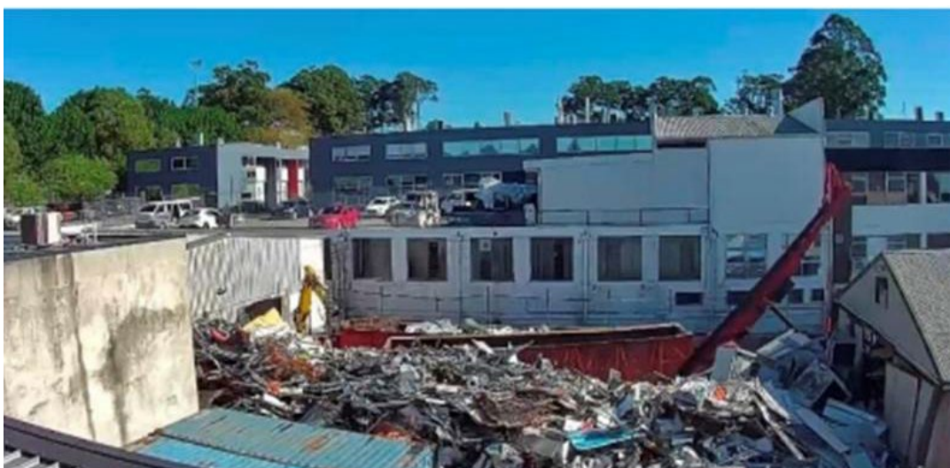
Figure 9: Empty skip bin for semi-trailer being delivered beside stock pile of scrap metal at 52 Buffalo Road
