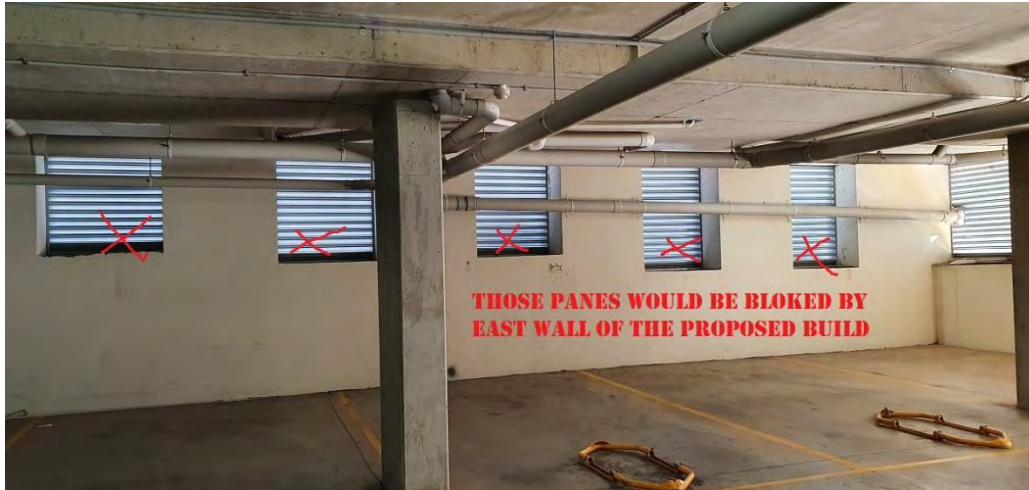
Figure 25: Photo provided by a submitter taken from within the at-grade car park of Nos. 10-12 Ethel Street showing 5 grates along the boundary shared with the subject site.
