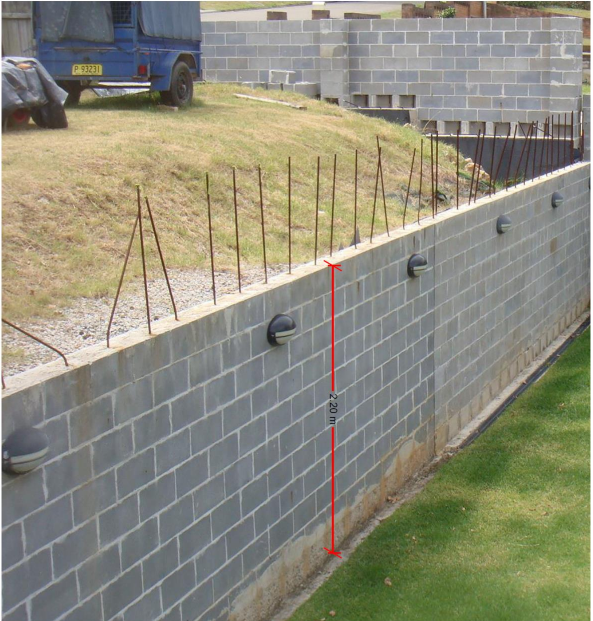
Photo showing the current status of the concrete block wall constructed in the middle of the site
