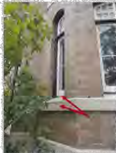
Figure 31a Paint peeling and cracked timber work and render ©2015 architects 2014
