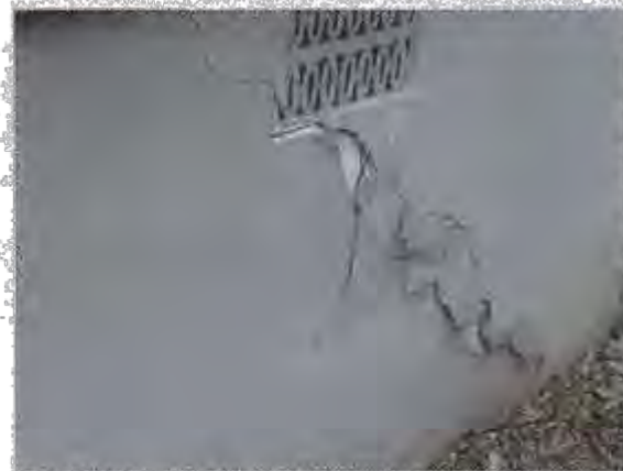
Figure 3.8 Damaged render to exterior base of Ben Leonard. Photo by Owner 2018
