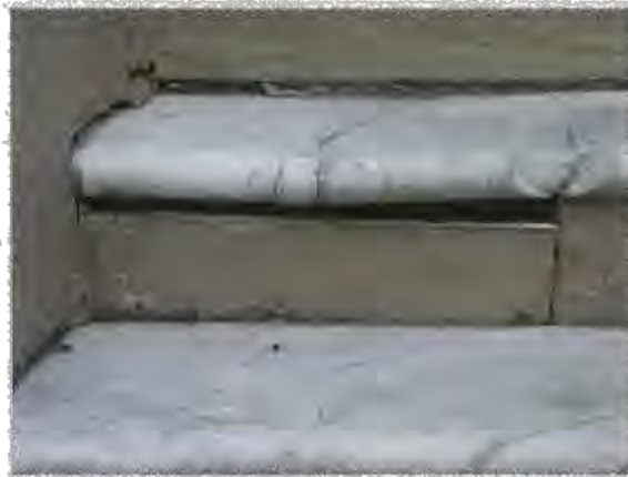
Figure 3.11 The north of entrance steps cracked and the foundation is sloping. Photo by Owner 2015
