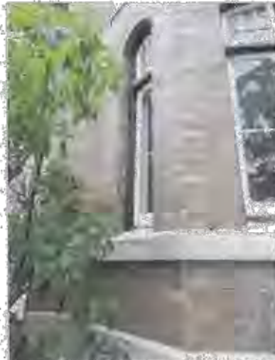
Figure 3.11 Paint is peeling and cracked on timber work (note 261) and render. OCP Architects 2014
