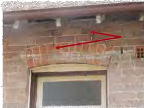
Figure 3.7 Cracking occurs in brickwork above openings of Ben Leonard. This example is from the kitchen wing. OCP Architects 2014.
