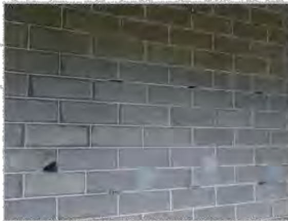
Figure 3.13 Signs of old pointing repairs are required. This photo is a detail from the front elevation of Ben Lomond. Photo by Owen 2015
