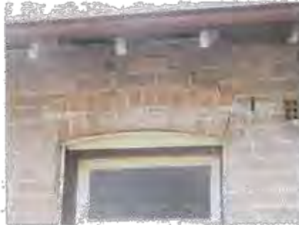
Figure 3.7 Cracking occurs in brickwork above openings. OCP Architects 2014
