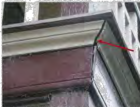
Figure 3.14 Timber casing of Ben Lomond requires repair. This example shows a detail of the top of the ground floor window. Photo by Owen 2015
