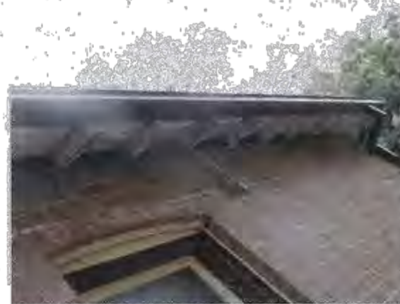
Figure 3.9 Timber rafters and soffit of Ben Leonard require repair and replacement. OCP Architects 2014
