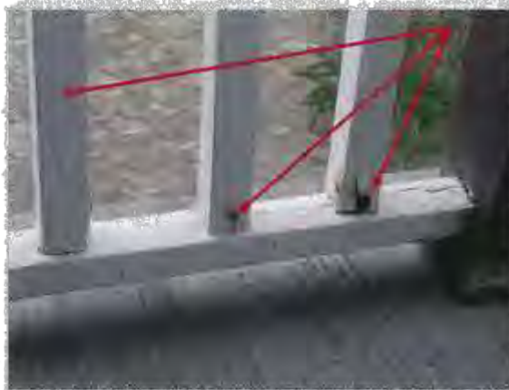
Figure 3.15 Damage to timber work and glazing of Ben Lomond. Furring strips require replacement as part of the repair work. Photo by Owen 2015
