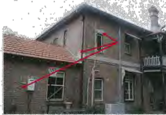
Figure 3.12 Poorly executed pointing requires replacement. This photo shows the north west elevation of Ben Leonard. Photo by Owner 2015
