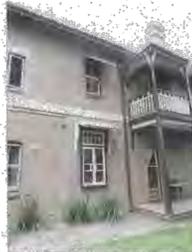
Figure 3.12 Painting to rear walls is poorly executed and requires replacement. OCP Architects 2014
