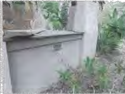
Figure 3.8 Damaged render to veranda base. OCP Architects 2014
