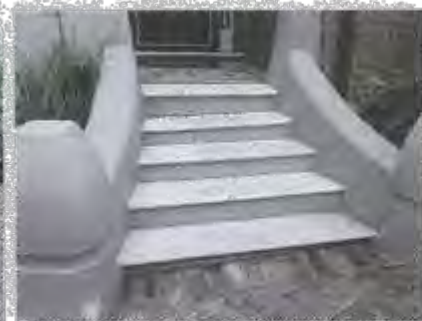
Figure 3.10 Marble of entrance stoop is cracked. The third second from the top is not fully supported and has dropped. OCP Architects 2014
