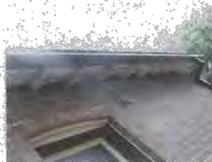
Figure 3.9 Timber soffits and eaves require repair and repainting. OCP Architects 2014
