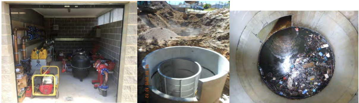
(Harvesting and UV treatment system, GPT being installed and collection 1 month after installation)
