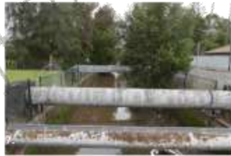
6 & 7. Morrison Bay Park is located on an infill site with an open concrete stormwater channel dividing the sportsfields. The retaining wall blocks have subsided significantly due to high rain fall events and high tides. There is limited pedestrian access across the channel.
