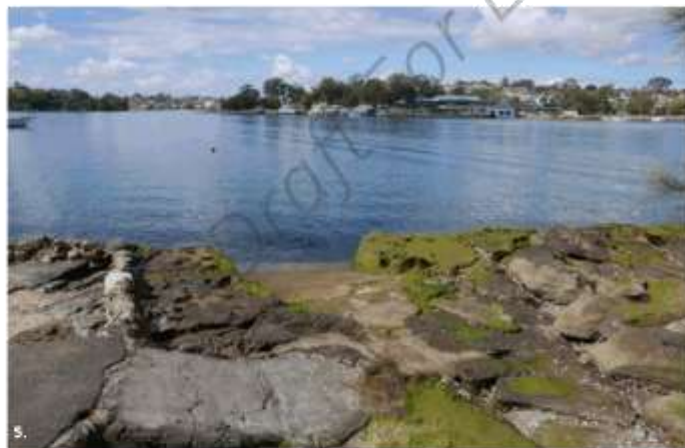
5. The boat ramp at Meditation Park is in poor condition
