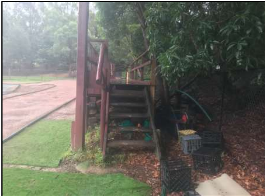
Fig 5. Eastern access to the platform. Note – tree butting up against rear and slope leading up to Epping Rd
