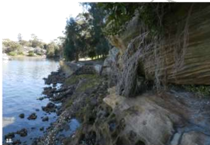
18. The seawall at Banjo Paterson Park is in poor condition. There is opportunity to provide continuous foreshore access as part of the upgrade to the seawall edge.
