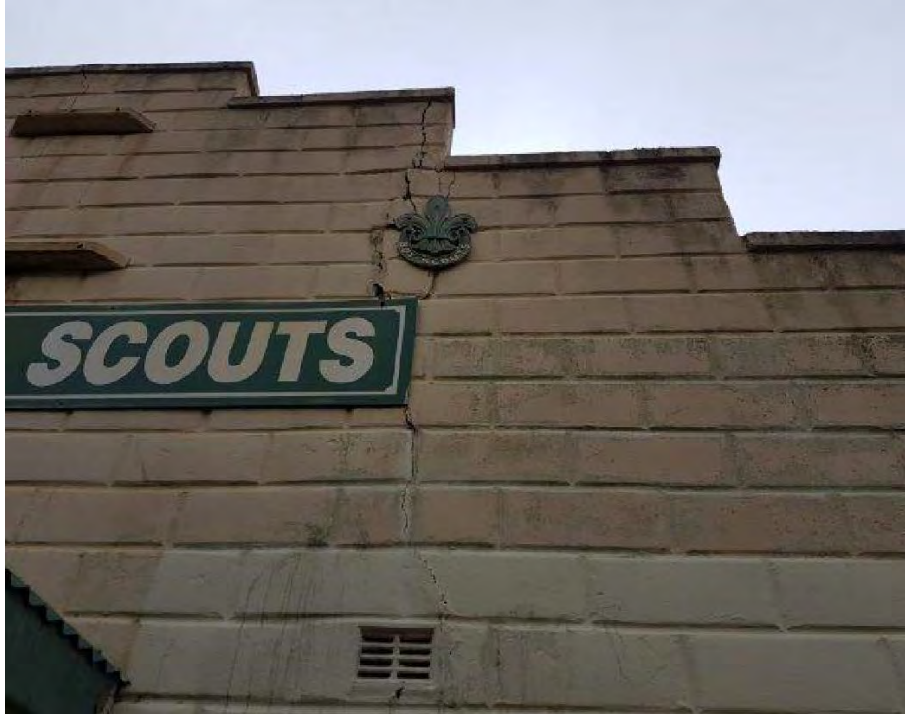
Photo 13 – Cracking forming through emblem
