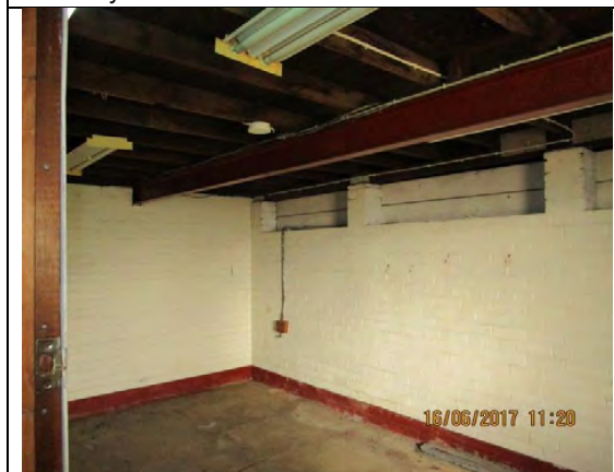
Lower Level Storage Room: Fire rate ceiling including steel beams and infill voids in masonry walls with fire grade plasterboard.
