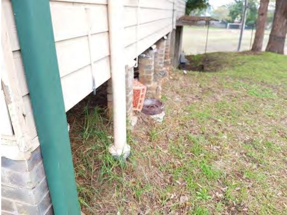
Photo 7 – A slight lean of the edge piers
