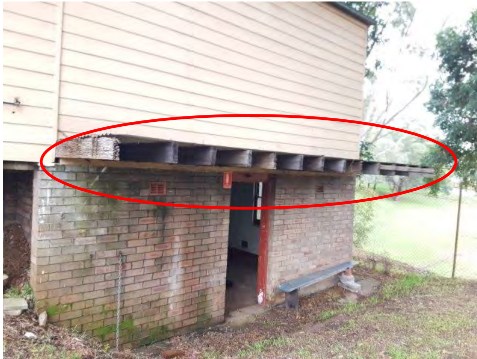
Photo 26 – heavy deterioration noted on storage awning.
