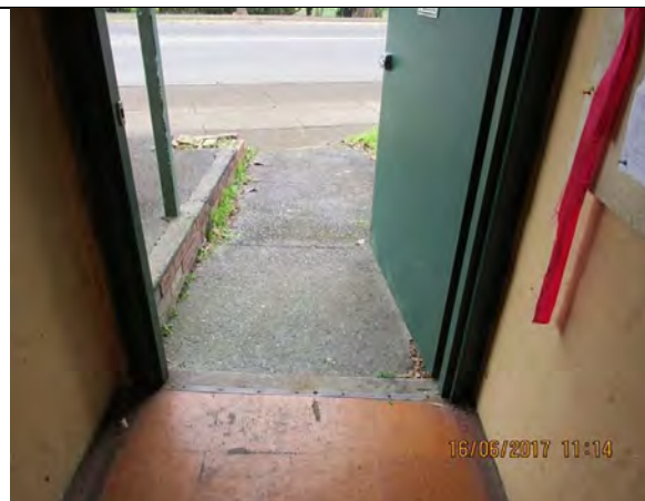
Front Door: View from internal corridor showing lack of latchside circulation space.
