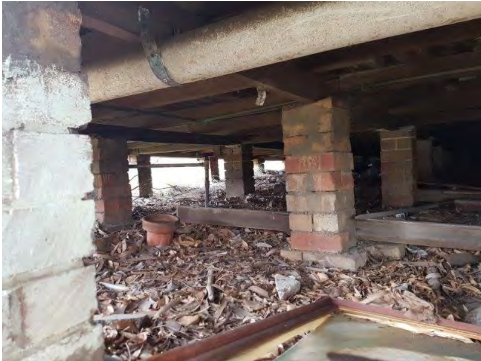
Photo 8 – General condition of existing bears & joists
