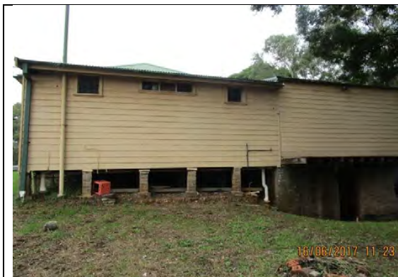
Rear of Scout Hall: Sufficient sub-floor ventilation and lower level storage room access door.
