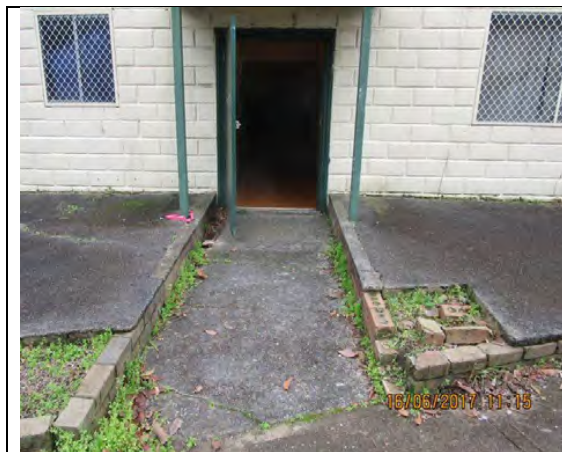
Front Door: Access to door via 1:40 path or 1:20 walkway in accordance with AS 1428.1-2009.
