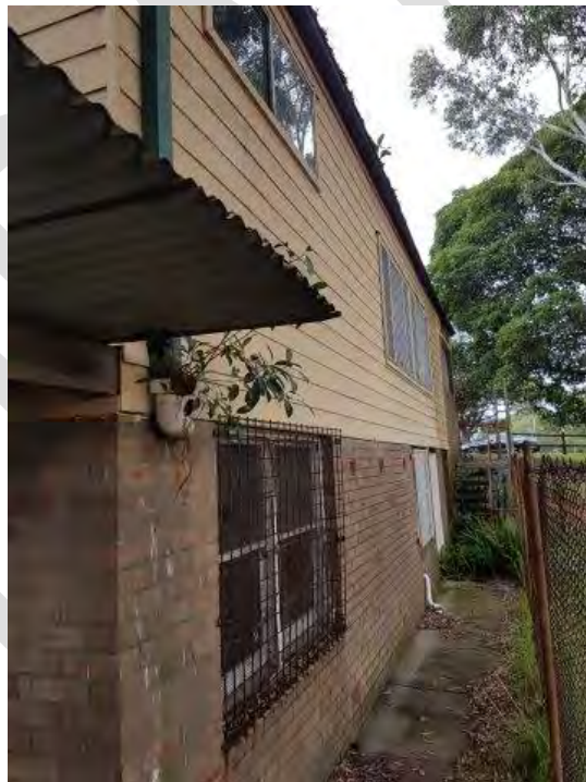
Photo 27 – Cracking noted on side paving.
