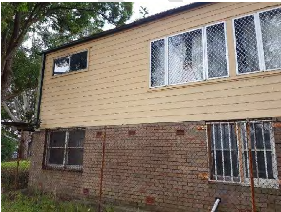
Photo 21 – General condition of external basement brick wall.
