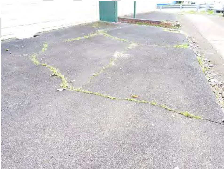
Photo 25 – Cracking noted on front paving.
