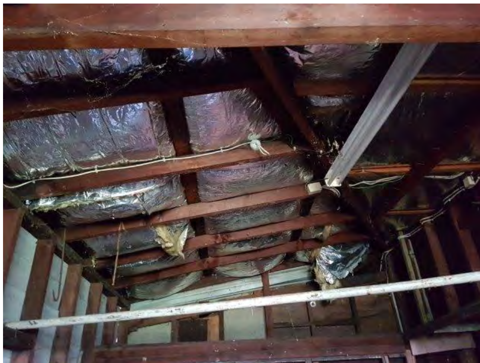
Photo 15 – General condition of roof members. Roof insulation exposed.
