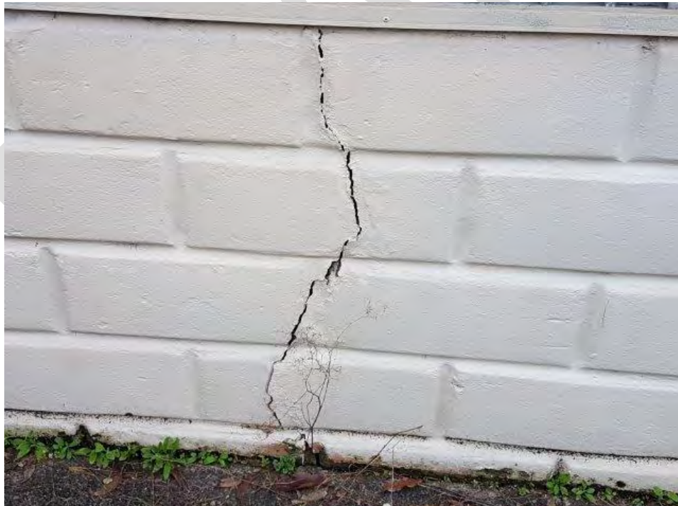
Photo 12 – Cracking below window opening
