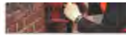
1. Rake out or cut slots into the horizontal mortar beds, a minimum of 500mm either side of the crack
