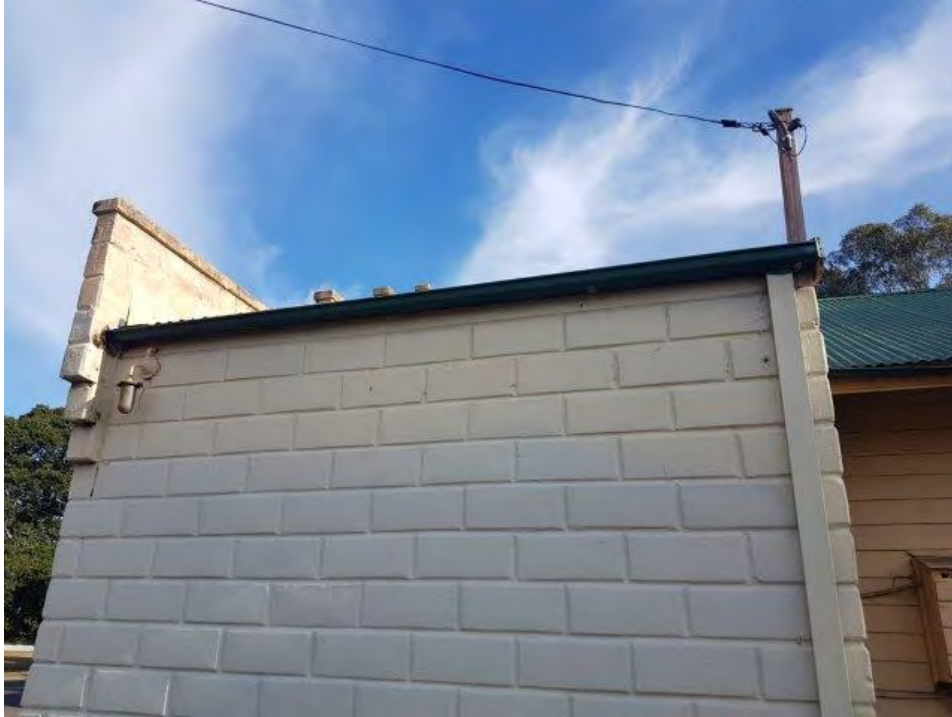
Photo 34 – leaning gutter noted
