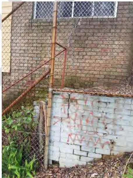
Photo 14 – settlement cracks noted on brick walls
