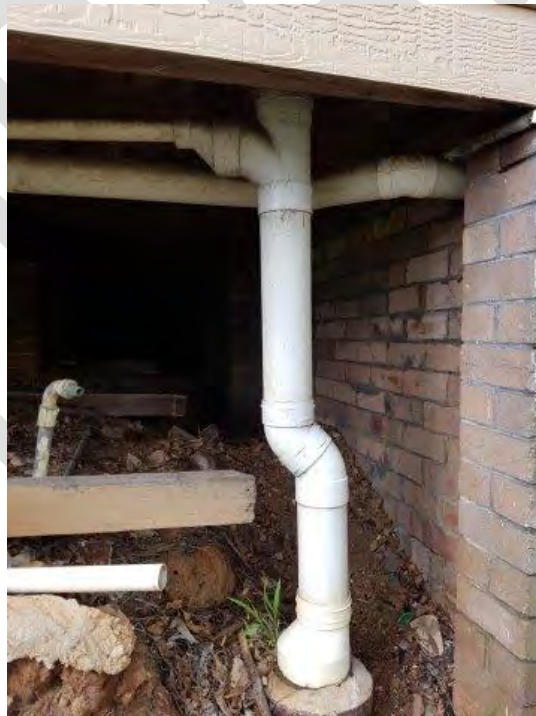
Photo 23 – No evidence of waterproofing observed.
