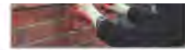
4. Using the HeliBar Insertion Tool, push one HeliBar into the grout to obtain good coverage
