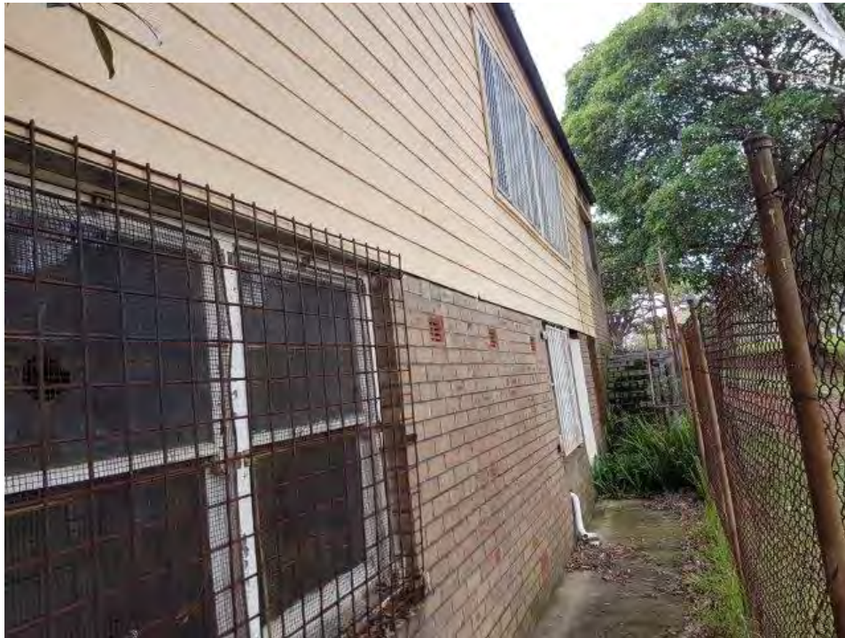
Photo 20 – General condition of external basement brick wall.
