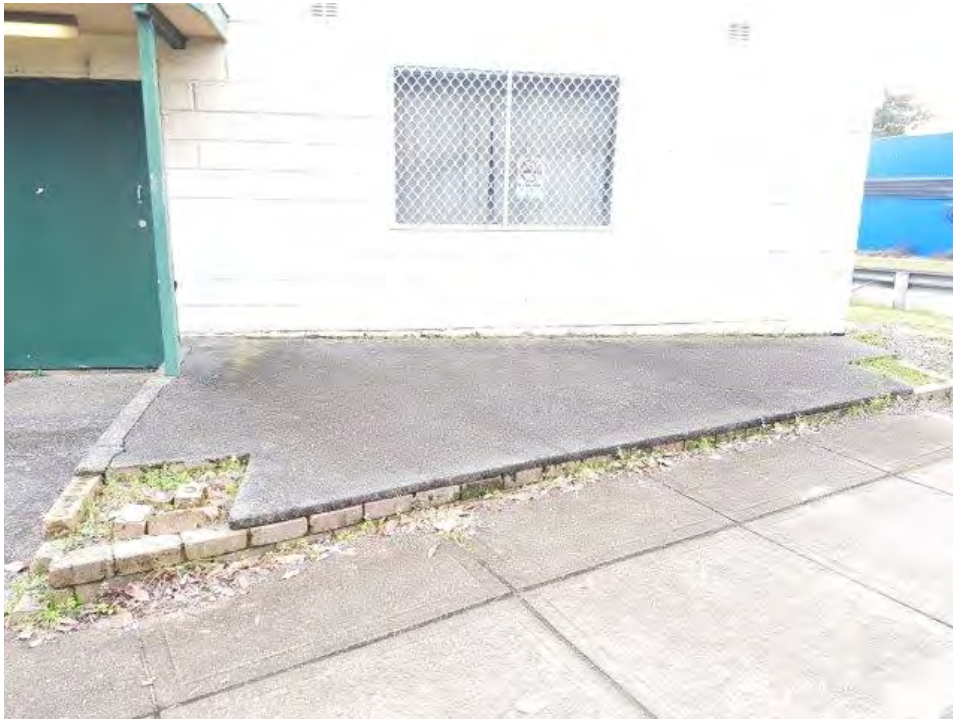
Photo 26 – Cracking noted on front paving.
