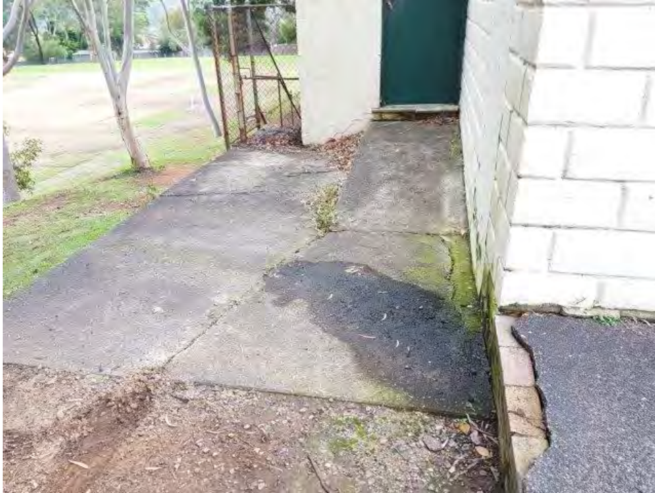
Photo 24 – Cracking noted on concrete paving.
