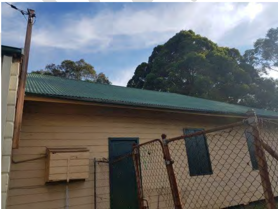
Photo 35 – leaning gutter noted
