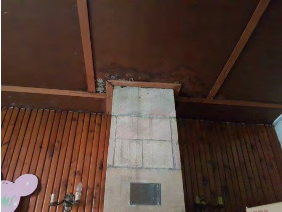
Photo 28 – moulding noted surrounding chimney.
