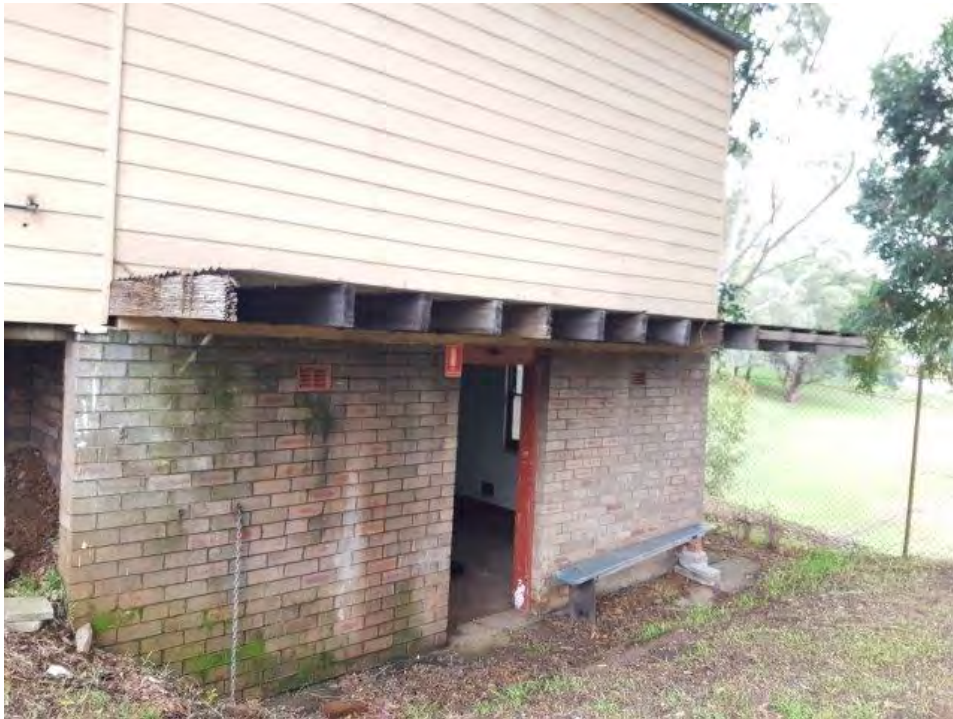
Photo 22 – General condition of external basement brick wall.
