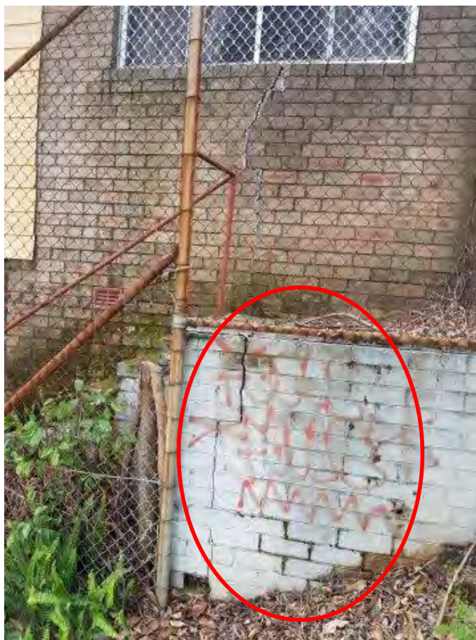
Photo 30 – dilapidated retaining wall to be replaced.
