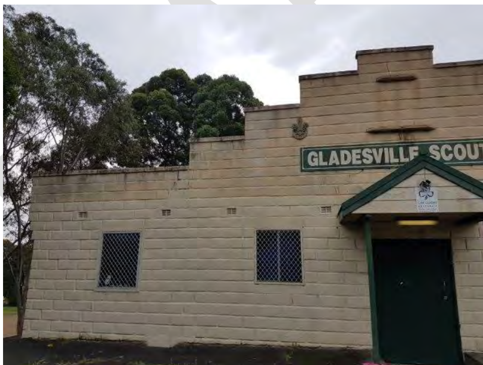
Photo 10 – Cracking noted on brick wall elevation
