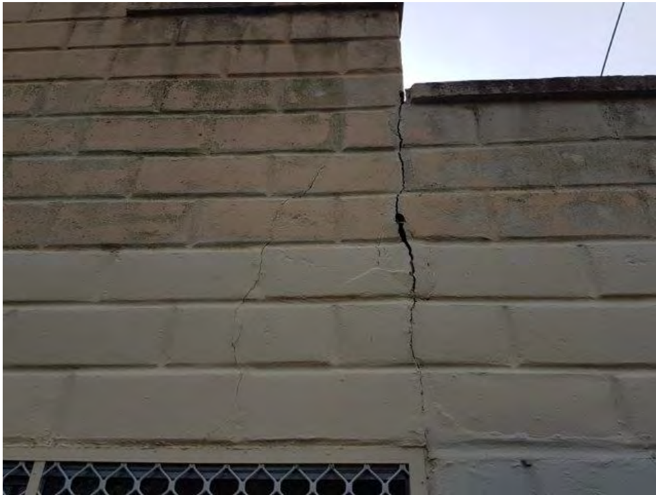
Photo 11 – Cracking noted forming from step-down
