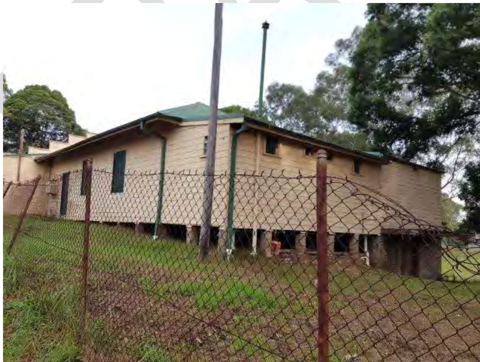
Photo 27 – Perimeter steel wire fence observed to be heavily corroded and leaning.
