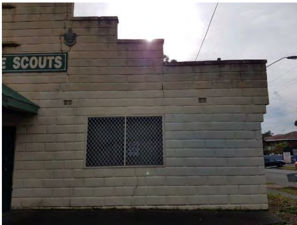
Photo 9 – Cracking noted on brick wall elevation
