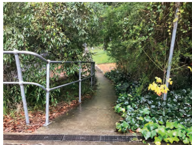
Non-compliant access from Epping Road
