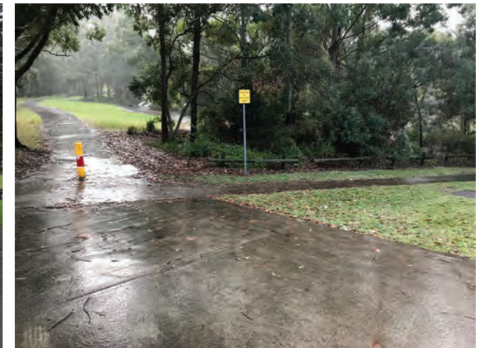
Drainage issues along Blenheim Road
