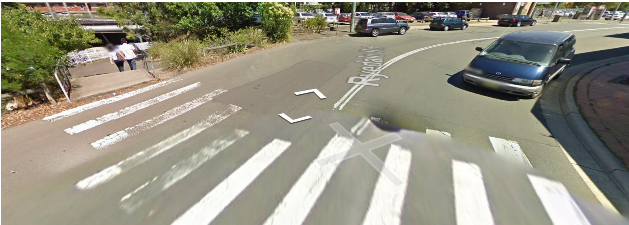
Figure E2: DDA Non-Compliant Pedestrian Crossing to be removed
