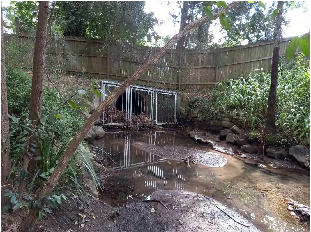
Figure 8 Piped waterway/ natural waterway – northern end
