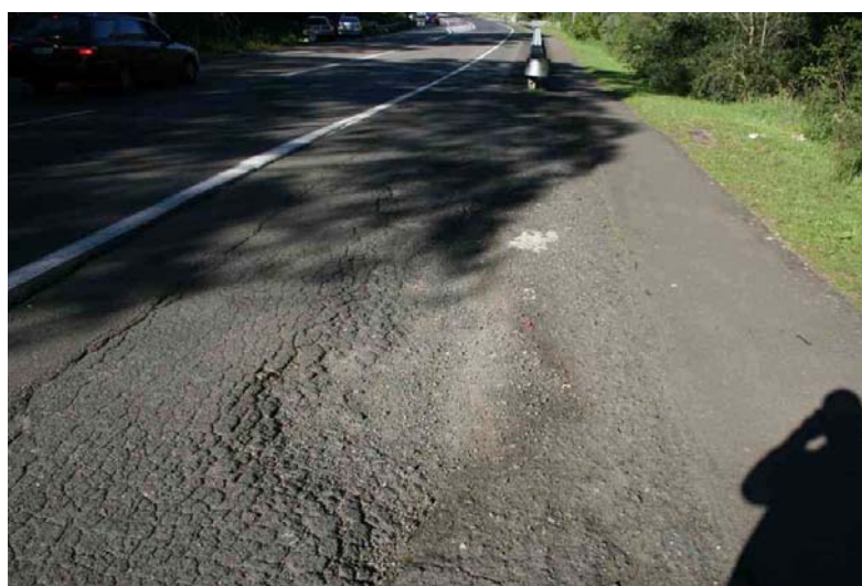
Figure 2.2: Example of an unsafe edge break.
