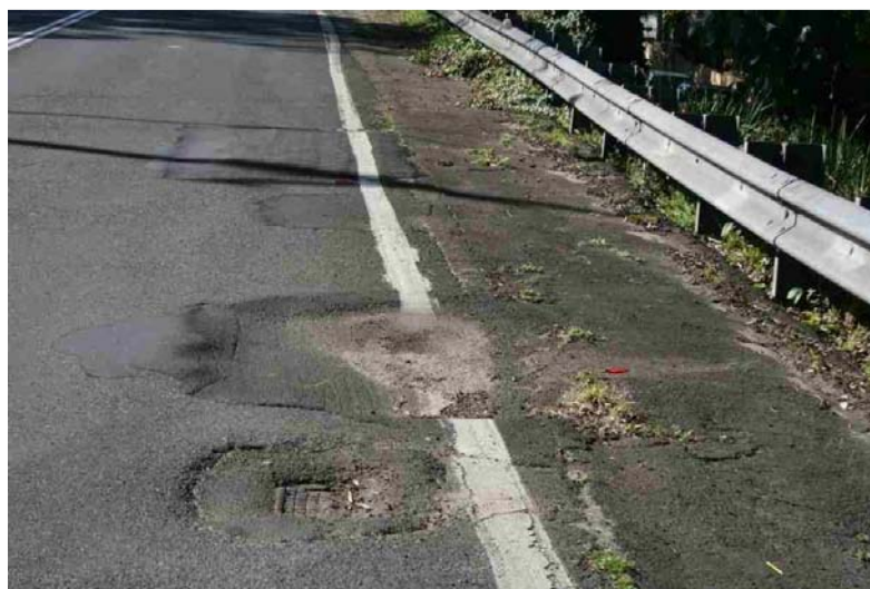
Figure 2.1: Example of failing pavement.
