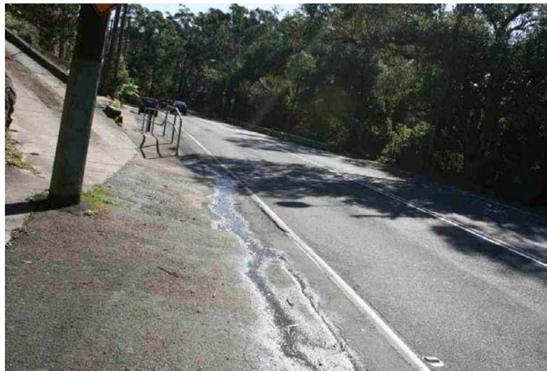
Figure 2.3: Example of irregular road surface.
