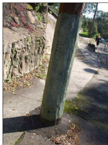
Photo 10: Light pole to be relocated (Plan 3 Appendix C ).
