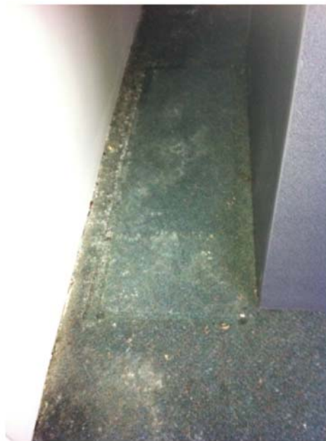
Photograph 3 Mould Growth on Area of Damp Carpet in Outreach Office.
