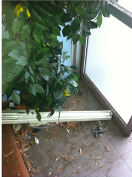
Photograph 4 Outreach Office – Leaves and Debris on Floor Near External Doors.
