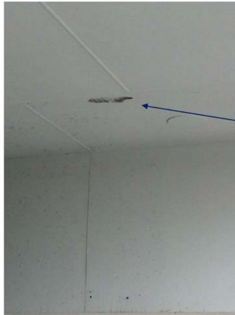
Black mould growth on underside of eaves.
