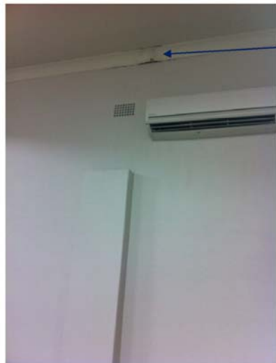
Photograph 2 Argyle Hall - Mould Growth Above Air Conditioning Unit.
