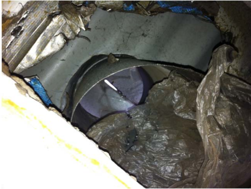
Photograph 6 Argyle Theatre – Close Up of Ventilation Pipe Allowing Water to Enter the Theatre During Rain.
