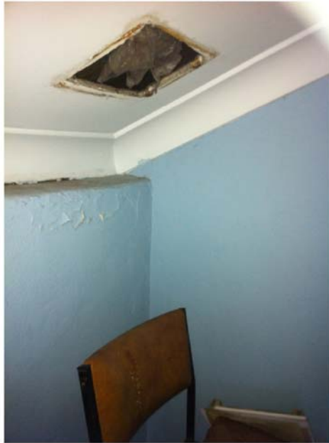
Photograph 5 Hole in Ceiling Cladding Where Water Was Entering Argyle Theatre.
