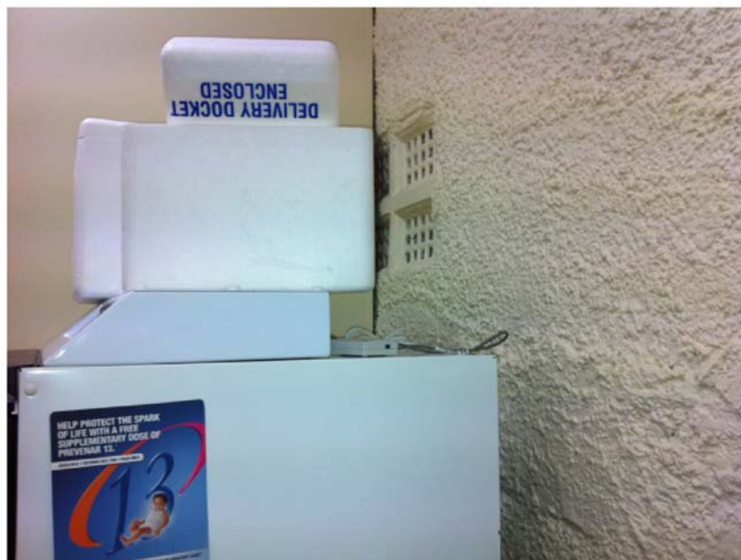
Photograph 1 Wall vents in Vaccine Store Room
