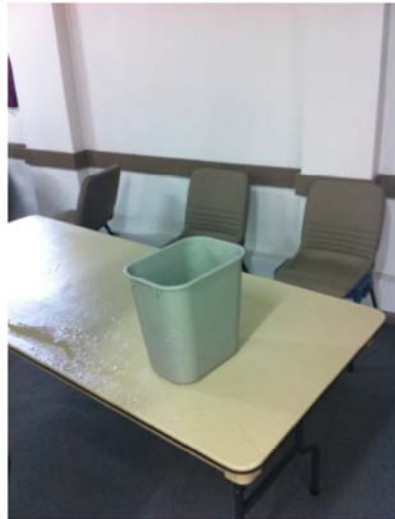
Photograph 1 Argyle Hall - Active Water Leak into (02/03/12)
