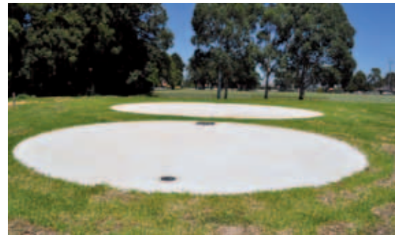
Epping Oval Stormwater Harvesting Project – Storage Tanks – Photo: Neil Keraunos.
