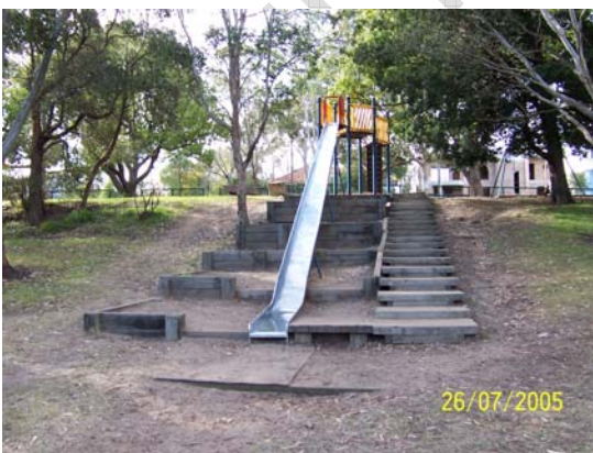
Playground equipment without any type of soft fall layer or other modern safety features. This equipment whilst still popular doesn't meet the latest safety standards and should be scheduled for removal and replacement.
