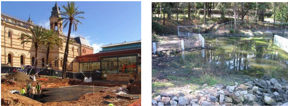
Figure 5: Stormwater storage being installed at the South Australian Museum (left), and stormwater harvesting pond at Barra Brui oval, St Ives (right).
