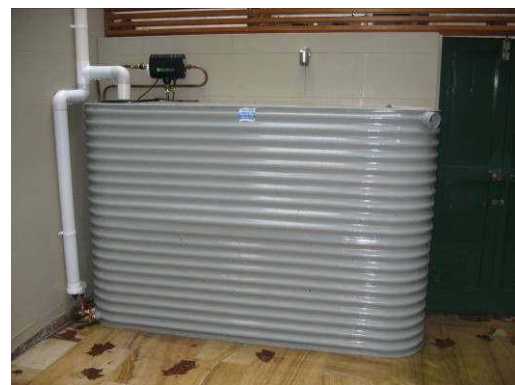
Figure 2 - Rainwater tank in residential property
