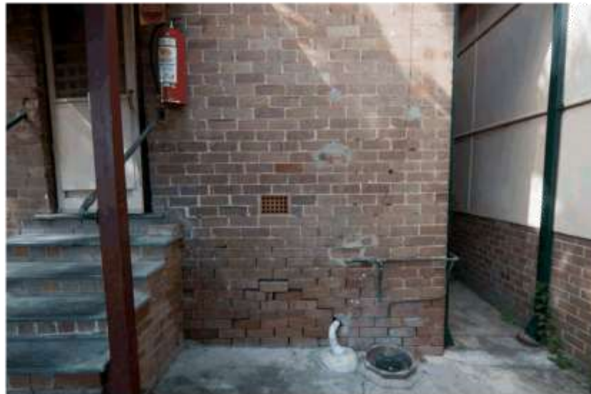
Figure 35: Detail at rear of the house showing damage to brickwork arising from issues with damp proofing
