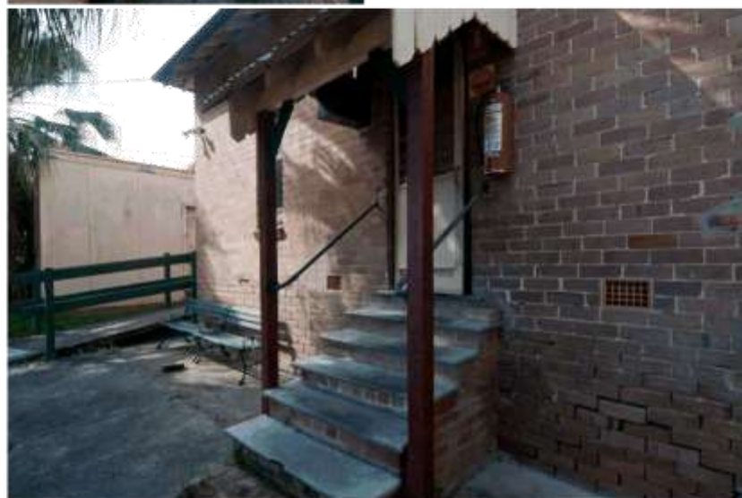
Figure 34: View along the rear wall of the original house showing damage arising from issues with damp proofing
