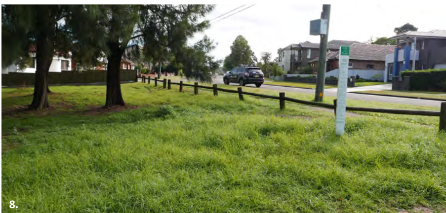
8. Boundary fencing at Melrose Park is dated.
