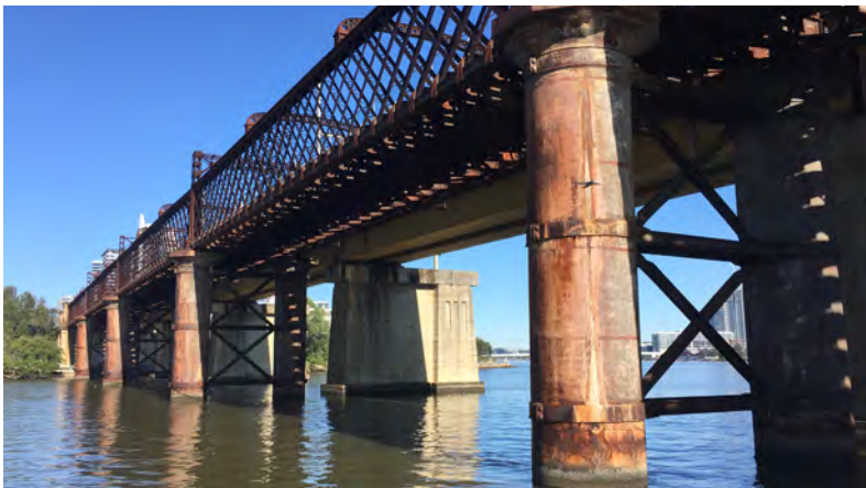
The Ryde Railway Bridge is a double lattice girder bridge that survives substantially in tact. In 1980 it was decommissioned as a rail bridge and is now used for shared access for bikes and pedestrians to link to other walking and cycling trails such as the Parramatta Valley Cycleway. It is listed on the NSW State Heritage Register.
