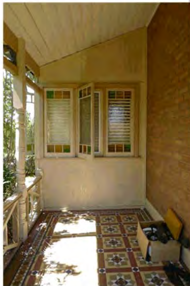
Figure 31: (Left) The northern elevation of the weatherboard clad ensuite built onto the eastern verandah, north of the central gabled bay.
