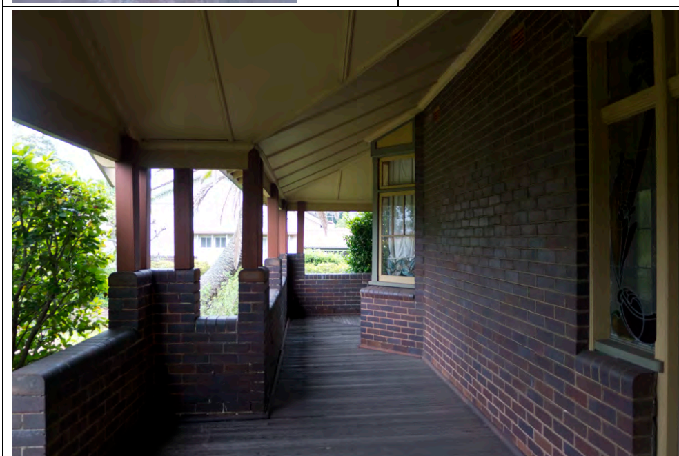
Figure 25: View along front verandah to the west, showing complex ceiling form and bay window.
