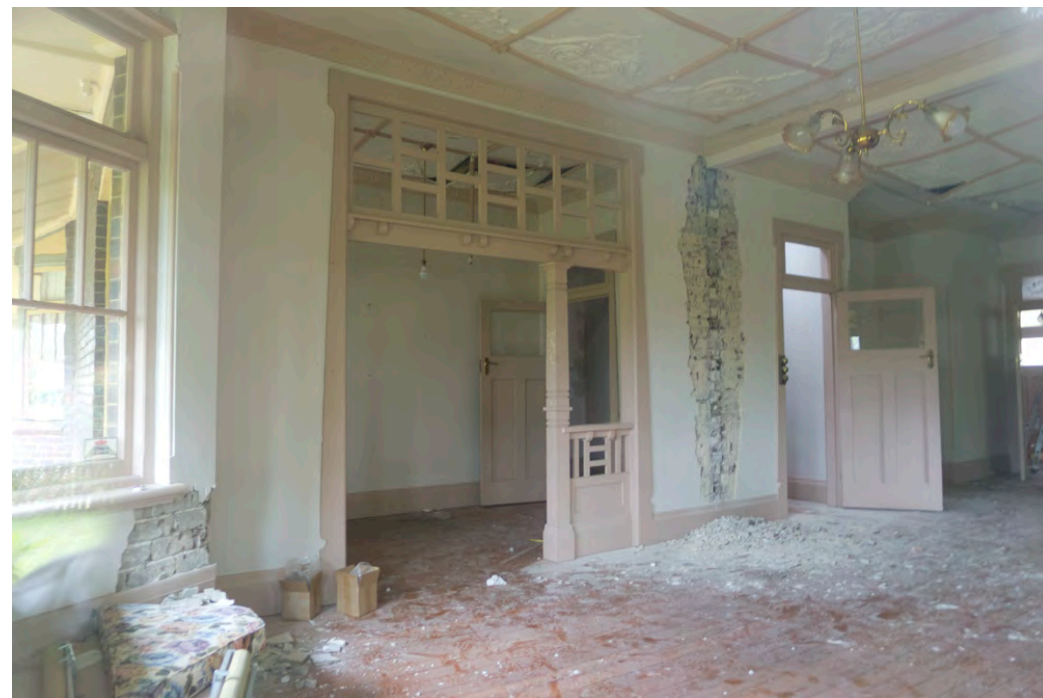
Figure 59: View of wall between loungeroom and hallway (foyer). Note the damage to the wall plaster is a result of illegal building works which occurred prior to the IHO on the site. Taken November 2018
