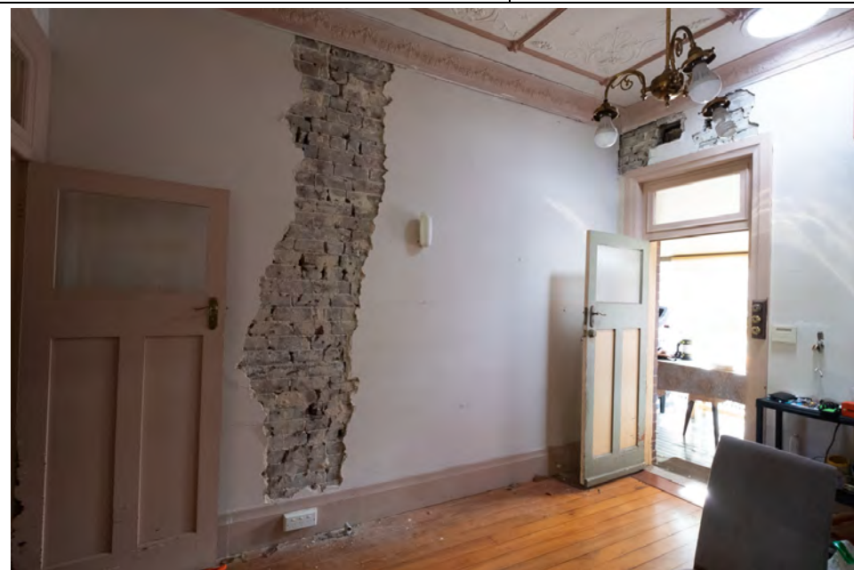
Figure 61: Breakfast room wall damage. May 2019.
