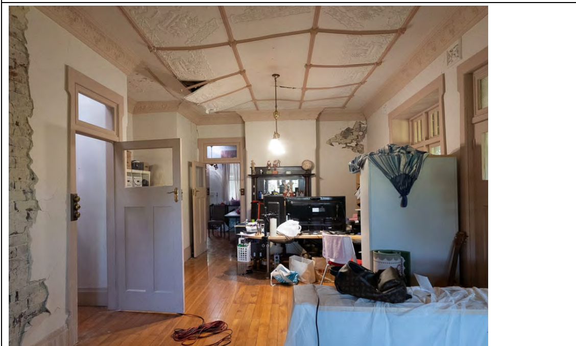
Figure 55: Same view of the dining room looking north towards the rear of the house, May 2019, noting ceiling and plasterwork damage.
