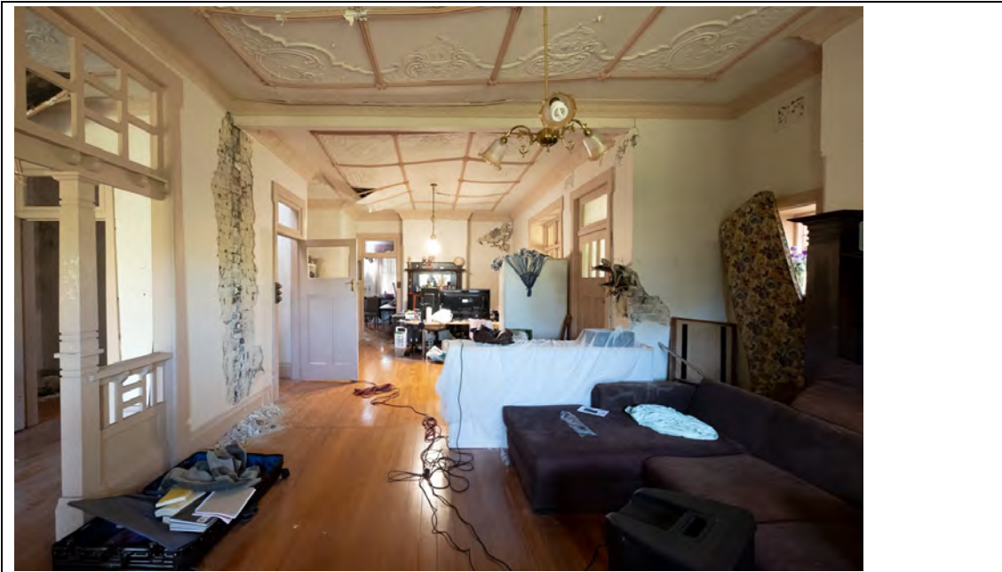
Figure 56: View of lounge room and dining room looking north, May 2019. Note damage to walls and collapsing ceilings
