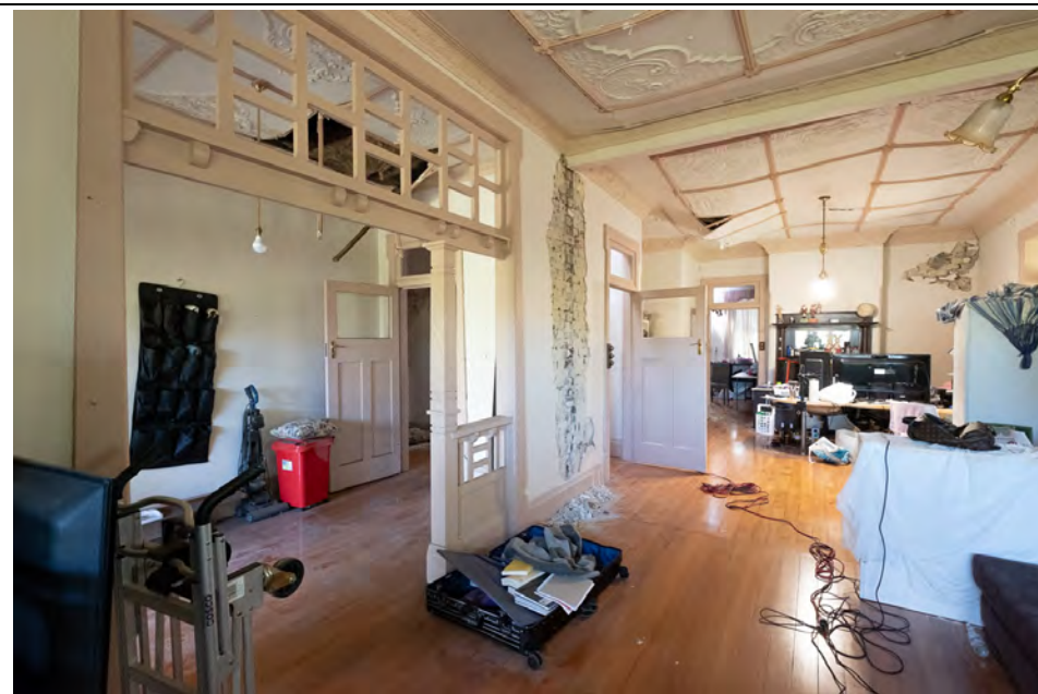
Figure 53: View of lounge room to hall, note wall damage and collapsing ceilings.
