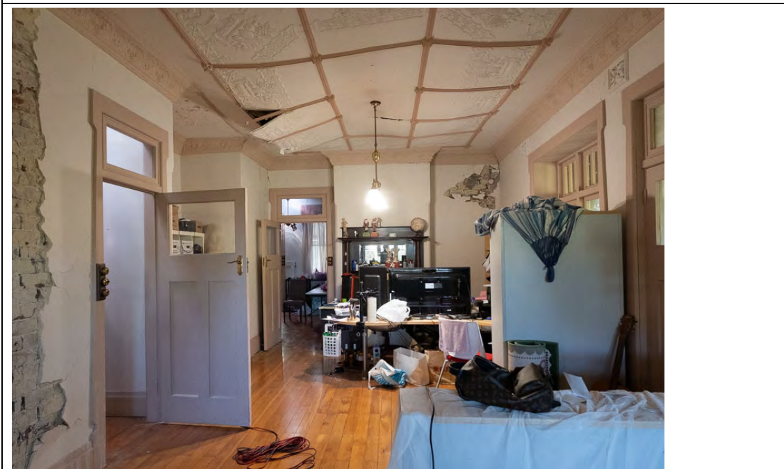
Figure 55: Same view of the dining room looking north towards the rear of the house, May 2019, noting ceiling and plasterwork damage.
