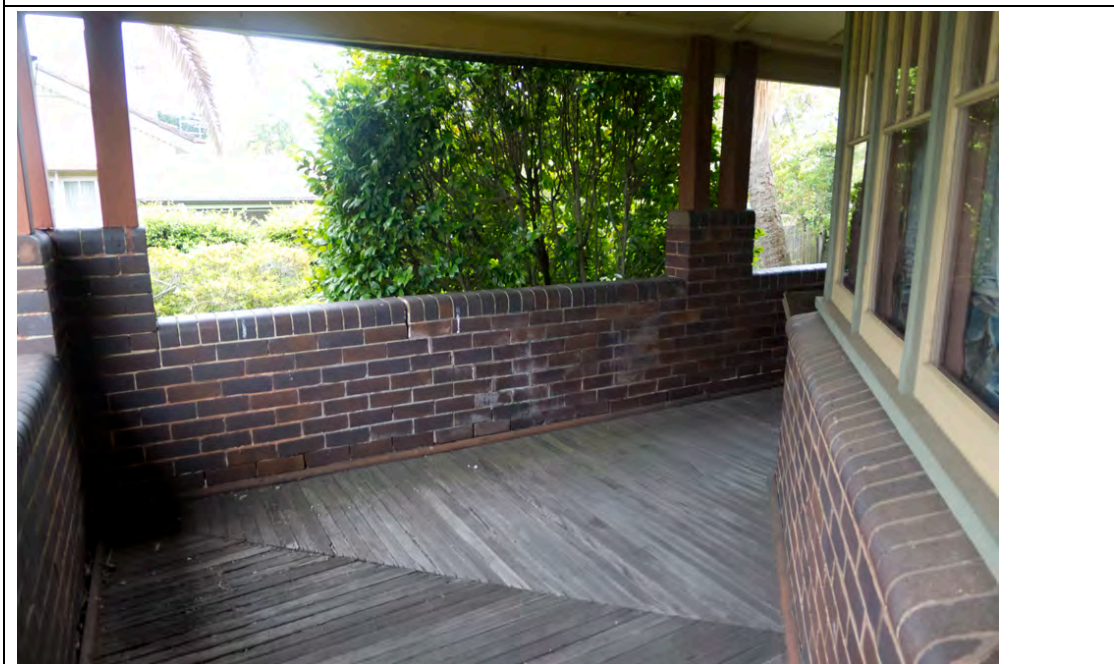
Figure 27: Detail of south-western corner of the return verandah showing brick balustrade, timber posts and timber verandah floor
