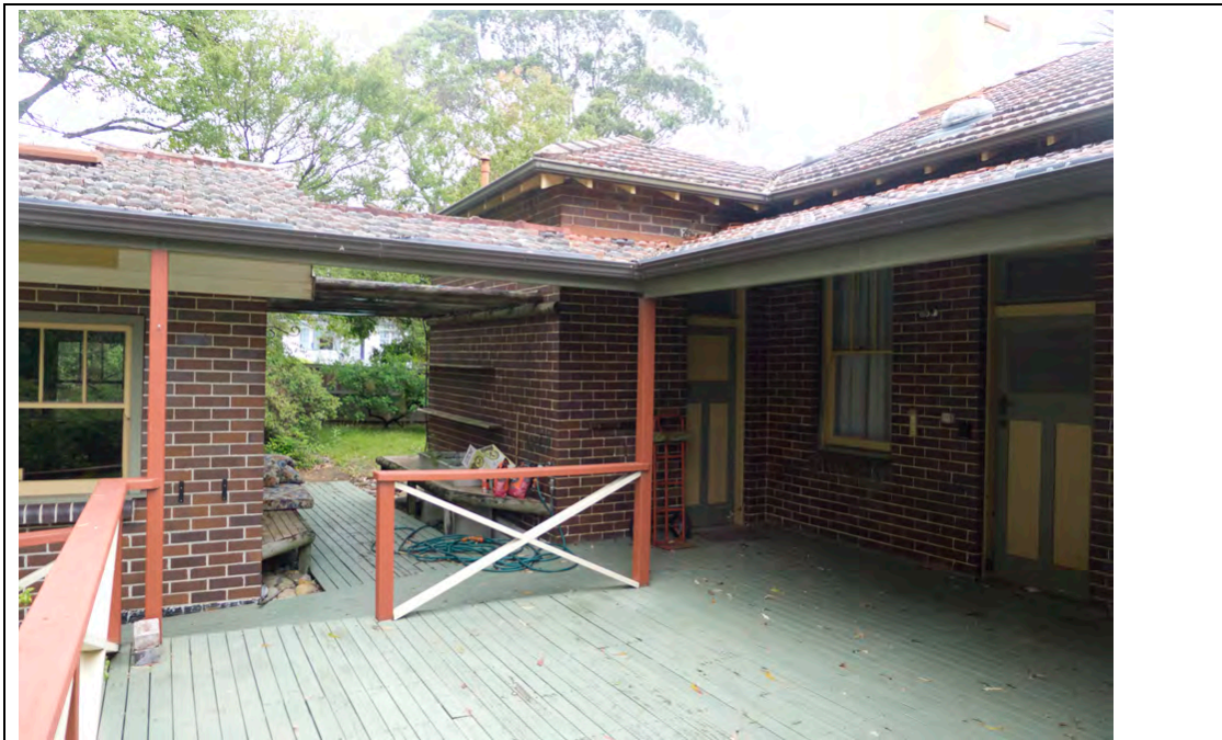
Figure 50: The eastern end of the rear (north elevation) of the house with the garage/workshop at left
