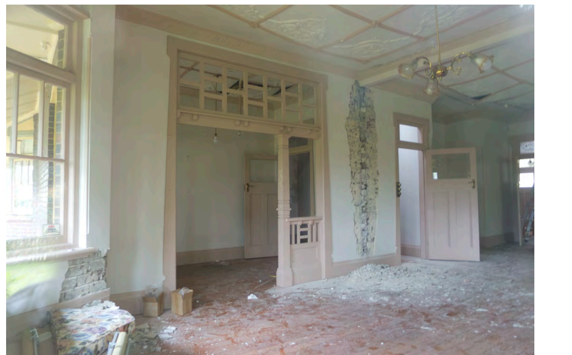
Figure 59: View of wall between loungeroom and hallway (foyer). Note the damage to the wall plaster is a result of illegal building works which occurred prior to the IHO on the site. Taken November 2018
