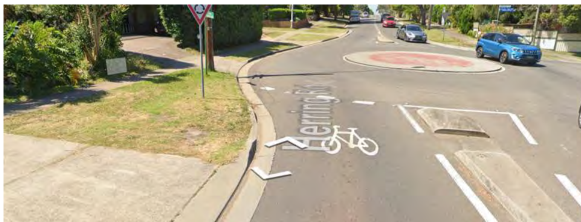
Figure 2: Missing Kerb Ramp on Herring Road
