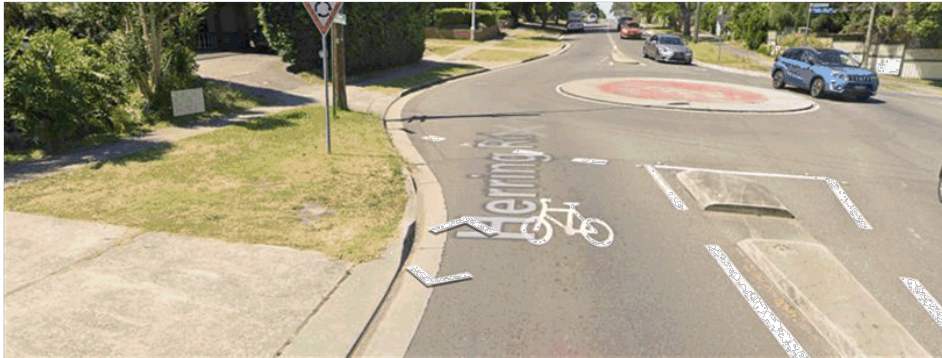
Figure 2: Missing Kerb Ramp on Herring Road
