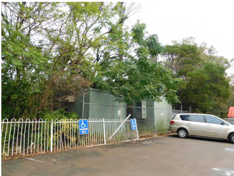
Figure 30: Electrical substations to the south of the club building. Note change of level beyond, where the south-eastern sports field is elevated.
