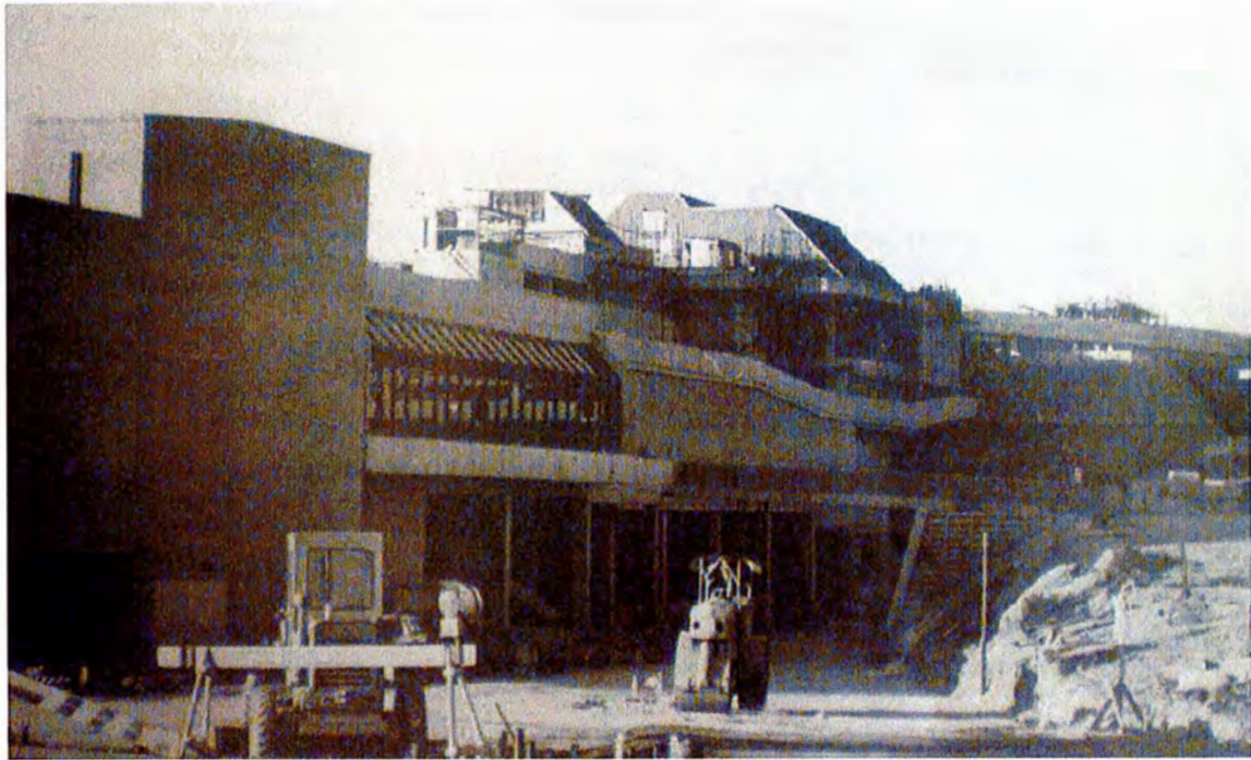
Figure 3.1 Macquarie Centre under construction, March 1981. (Source: Coles Myer Archive, Macquarie Centre newsletter, Vol. 1, No. 1, State Library Victoria)
