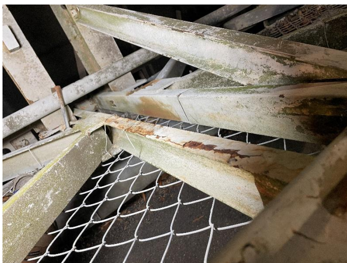
Figure 17 Coating delamination on posts and diagonal bracings
