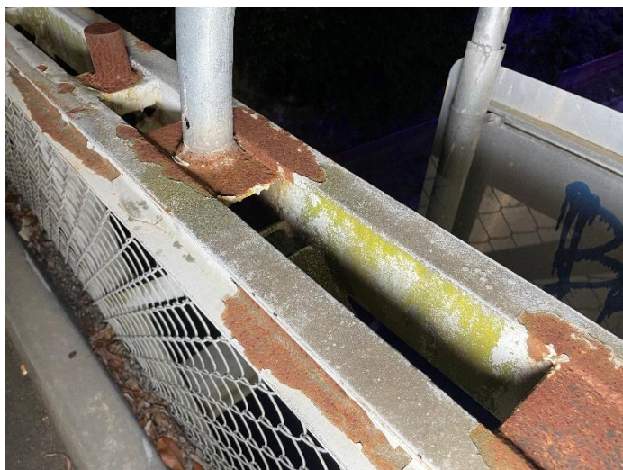
Figure 15 Coating delamination and surface rust
