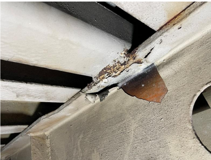
Figure 3- Flaking defect on transom
