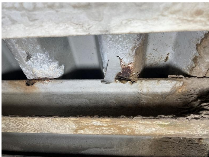
Figure 11 Corrosion between girders and trough decking sheets
