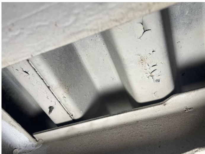
Figure 13 Delamination between paint and galvanised substrate
