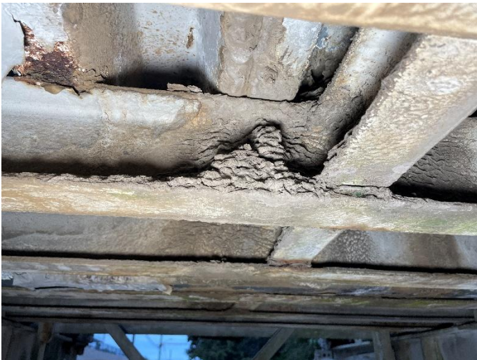
Figure 7 Accumulation of contamination
