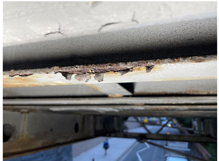
Figure 8 Coating delamination and corrosion on edges
