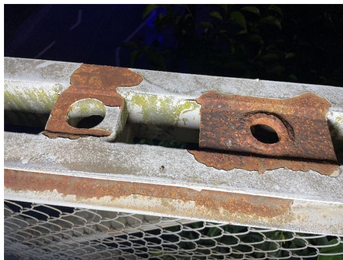
Figure 16 Coating delamination and surface rust
