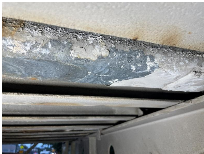
Figure 10 Poor adhesion between paint and galvanised coating
