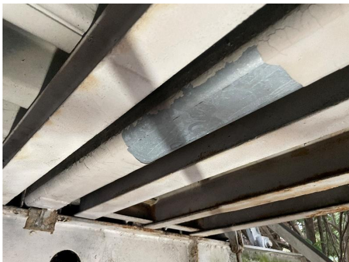
Figure 9 Delaminated paint from galvanised substrate
