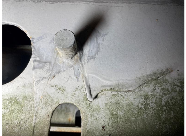
Figure 6 Evidence of poor coating touch-ups
