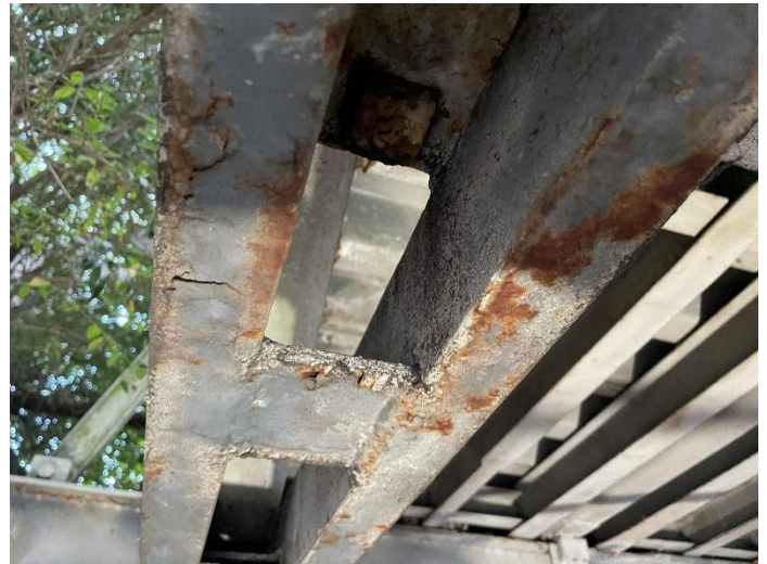
Figure 2- Coating delamination and surface rust on bottom chord
