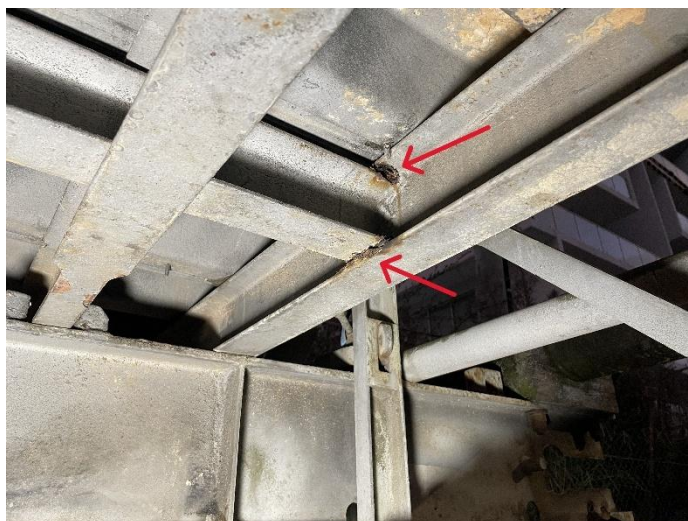
Figure 12 Corrosion on welds
