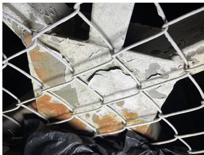
Figure 18 Coating delamination on connection plate
