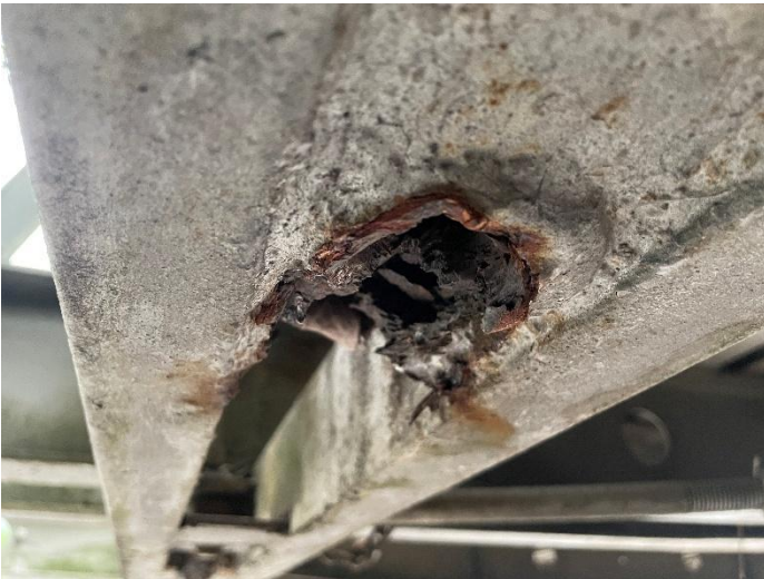
Figure 1- Heavy spot corrosion on bottom chord
