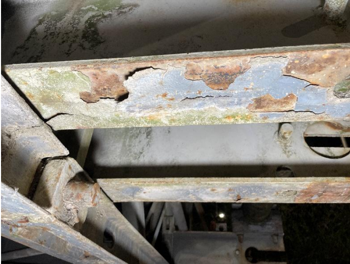
Figure 5 Coating flaking and surface rust
