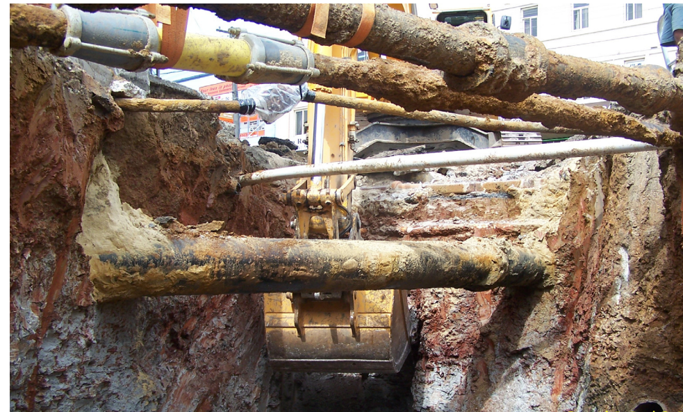
This photograph illustrates the skill and care required by the team while working around the intricate network of existing underground services.
