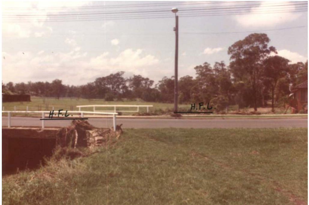
Photo A1.7: Debris deposited at Kent Road culvert crossing, looking downstream. (Ryde City Council photo 'S23')
