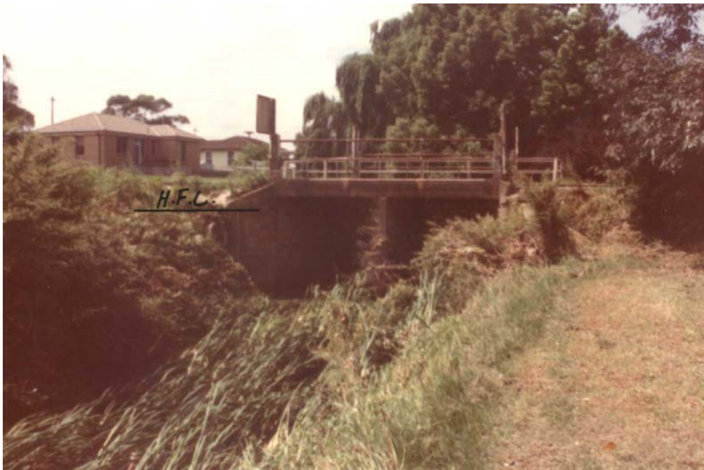
Photo A1.12: Photo taken of Bridge Road bridge, looking downstream from Santa Rosa Park.
