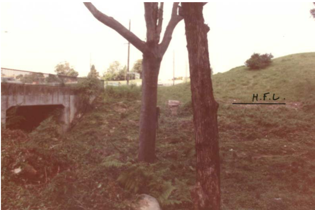
Photo A1.6: Debris line on southern bank of Shrimptons Creek just upstream of Epping Road bridge.
