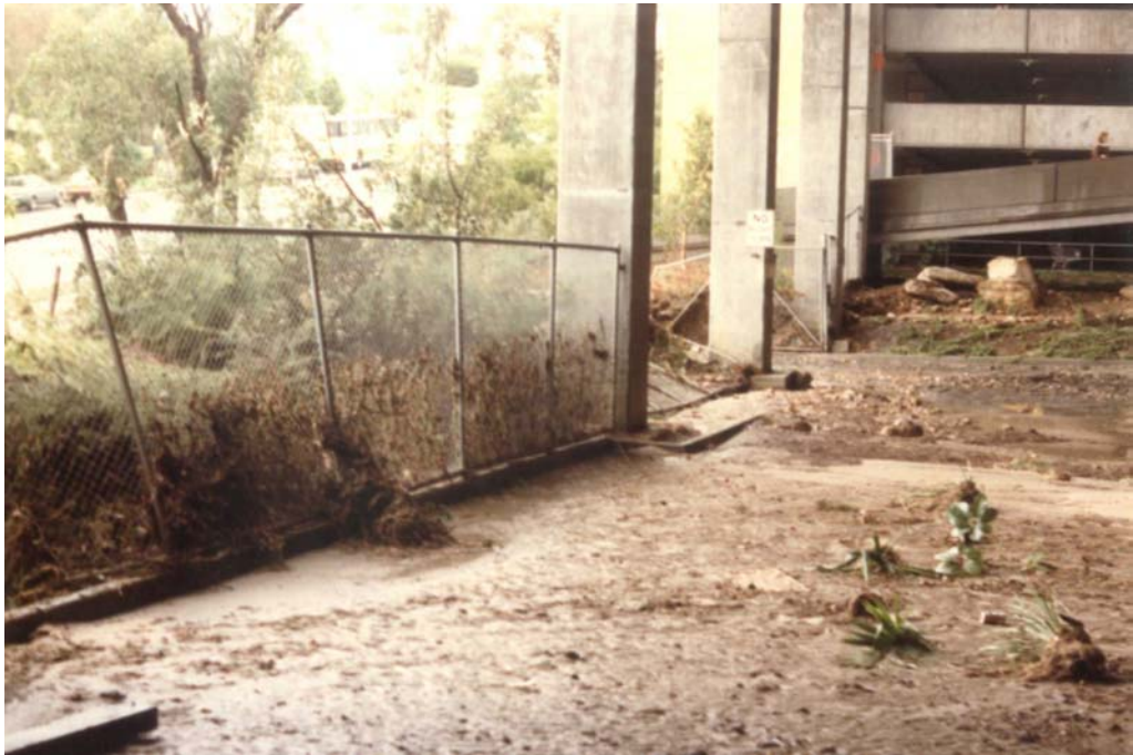
Photo A1.3: Debris caught on fence at Macquarie Shopping Centre's frontage to Talavera Road. (Ryde City Council photo 'S5')
