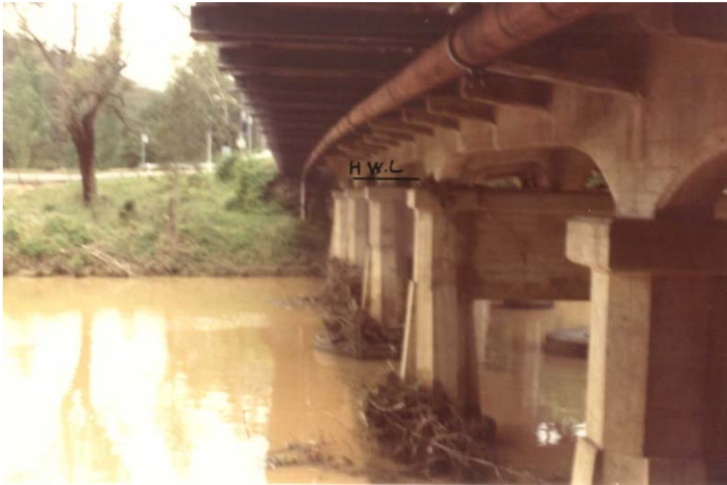
Photo A1.1: Fullers Bridge across Lane Cove River, looking east, showing debris deposited on bridge columns.
