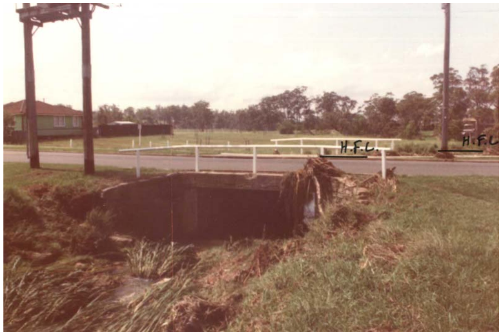
Photo A1.8: Debris deposited at Kent Road culvert crossing, looking downstream. (Ryde City Council photo 'S24')
