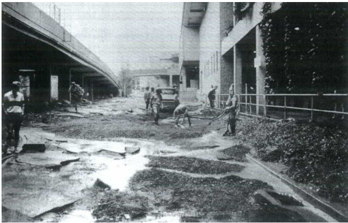
g. November 1984, Macquarie Shopping Centre, Macquarie Park. Shows damaged internal road as asphalt was stripped away.
