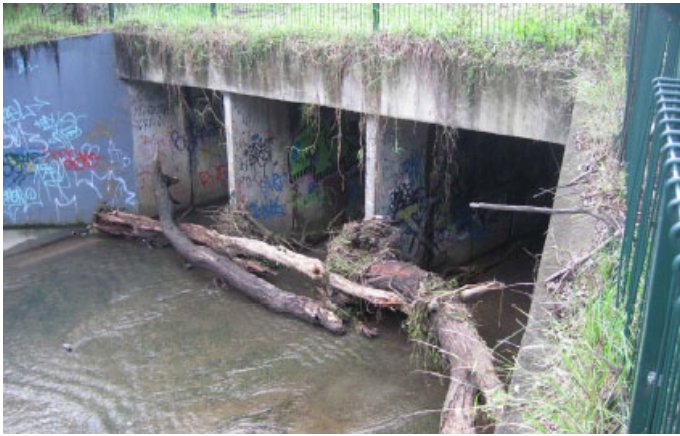
k. February 2010, blockage at the Shrimptons Creek culvert, Waterloo Road, Macquarie Park.
