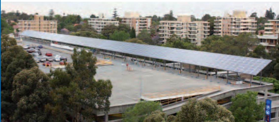
Stage 2 Solar Farm in Chatswood' Albert Street car park.
