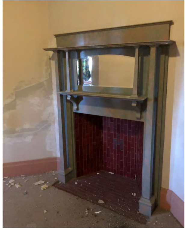
Figure 16 – View of fireplace in front bedroom with evidence of major cracks to the left Source: Urbis
