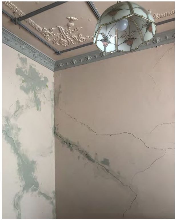
Figure 18 – View of major cracks previously patched Source: Cheng Yang 2019
