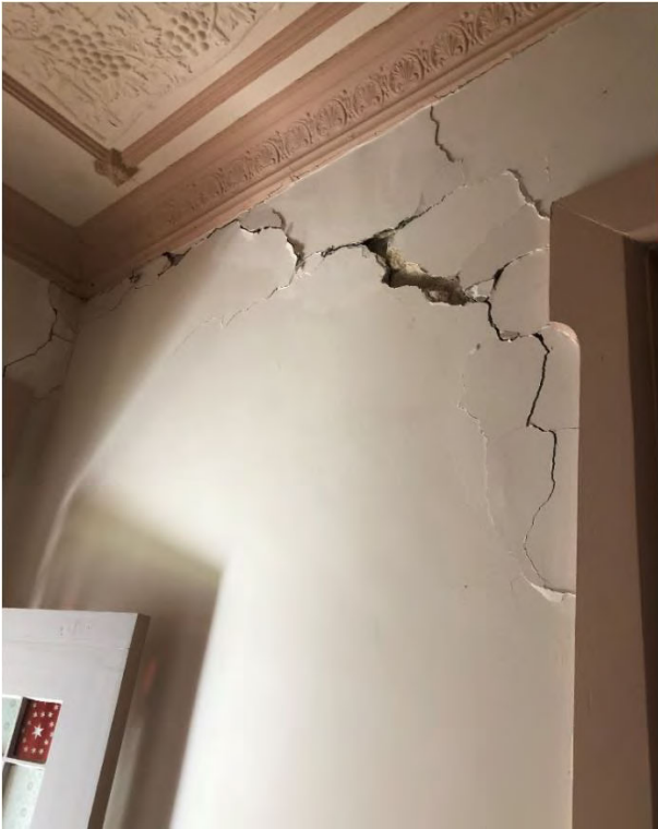
Figure 15 – View of typical crack in masonry wall Source: Urbis
