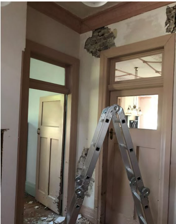
Figure 17 – View of cracks above door and drummy render Source: Urbis
