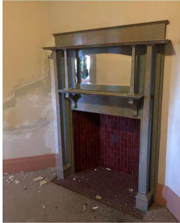
Figure 16 – View of fireplace in front bedroom with evidence of major cracks to the left Source: Urbis
