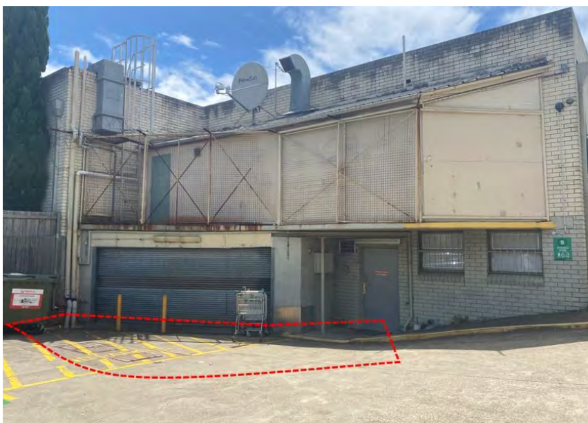
Figure 19: Location of depression identified in red & exhibits an existing ground level ranging from RL 47.38 to RL 47.79. Source: CPS – Site Inspection, 16 January 2023
